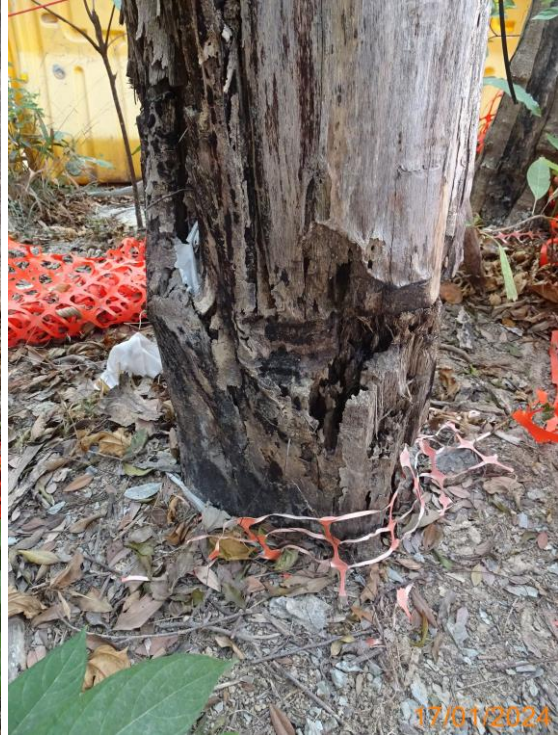
10: U041_Wood damaged by termite
