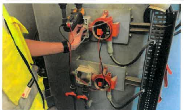
0ppm Calibration for Outlet H2S Sensor
