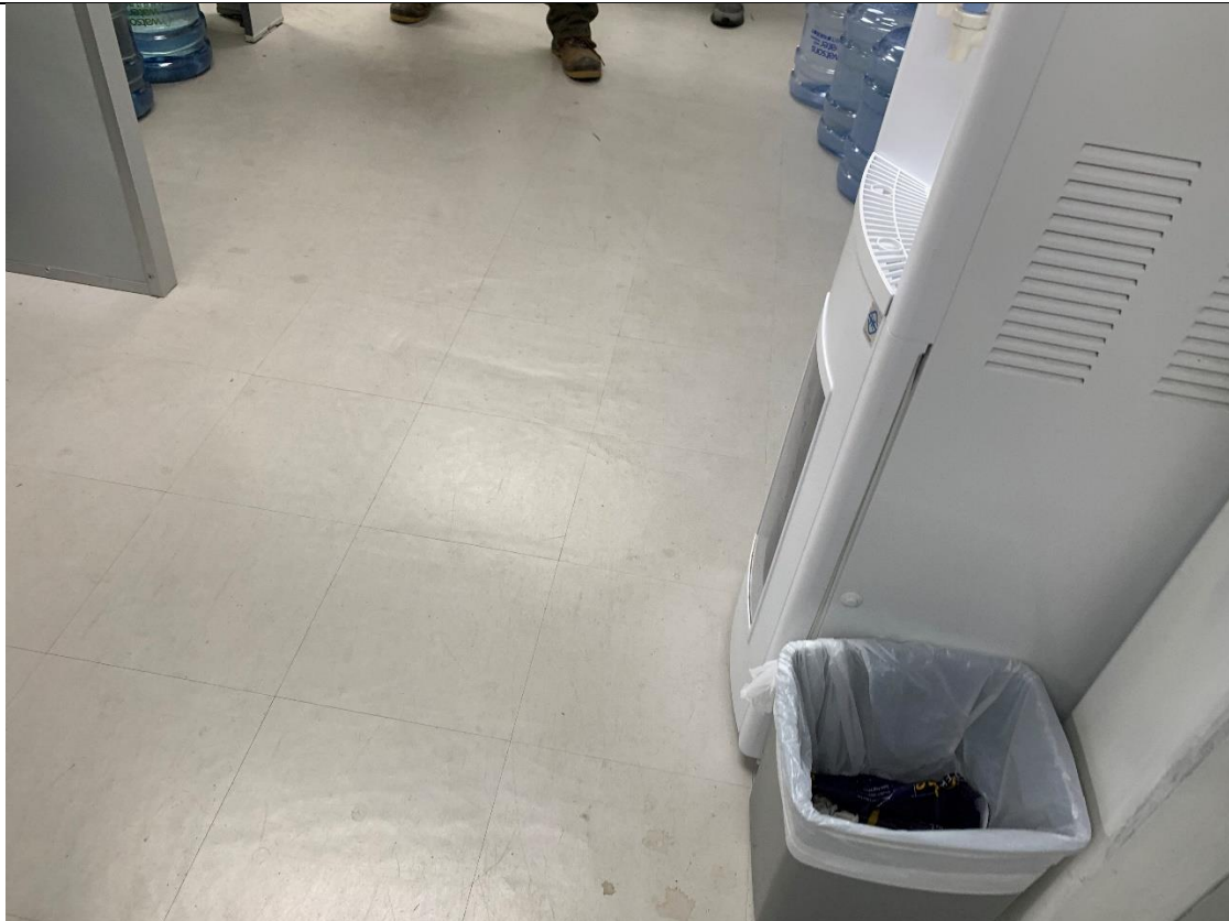
Photo 29 – Floor Condition of the Site Office, G/F
