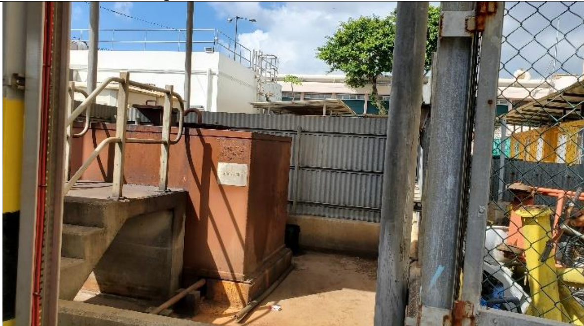
Photo 6 – 4000L chemical waste collecting tank
