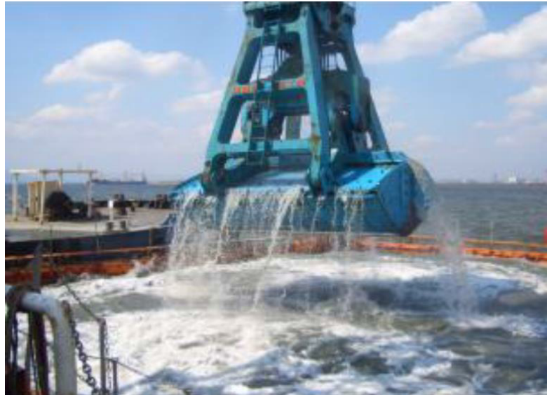
The silt curtain separates the dredging zone from the nearby waters to minimize water pollution nuisance
