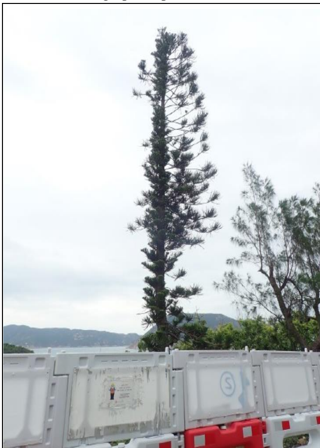
Plate 2. Photographic updates of the three retained trees that close to construction activities.
