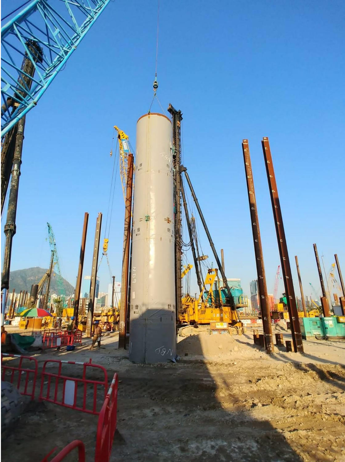
1. Noise barrier for percussive piling had been used to reduce the noise nuisance to sensitive receivers.
