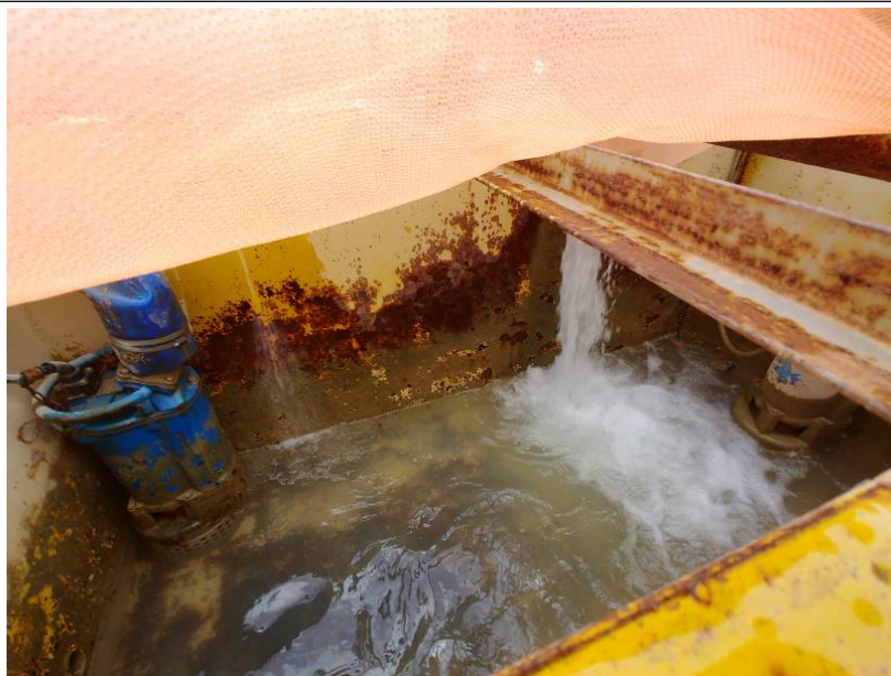
Photo 4b: Effluent Tank at Wastewater Treatment Plant (16 September 2020)
