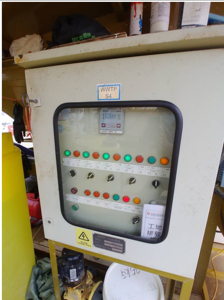
Photo 4a: pH value at Wastewater Treatment Plant (16 September 2020)
