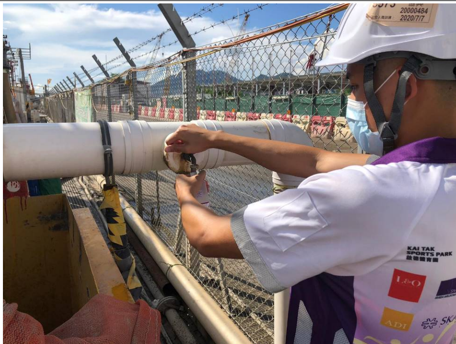
Photo 6a: Regular Sampling at Wastewater Treatment Tank Discharge
