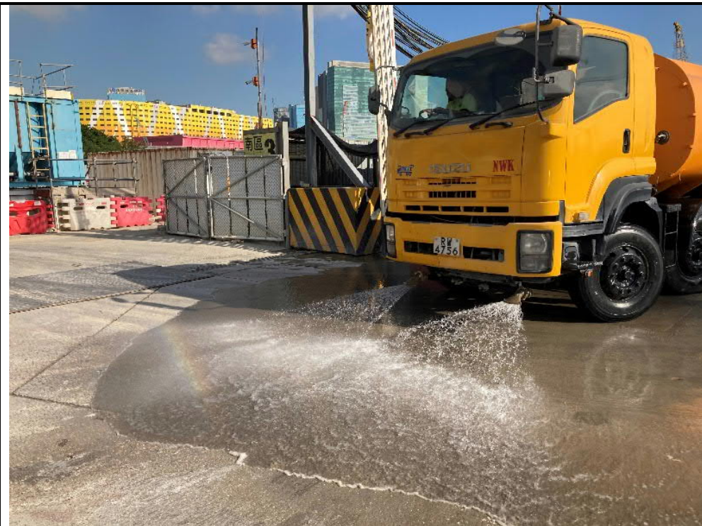
Photo 5: Water spraying truck routinely washes the main haul road and public road to maintain wet surface
