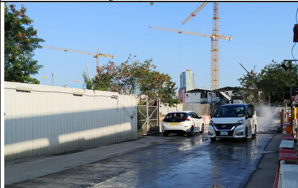
Photo 2: Wheel washing facilities had been implemented for the passage of construction vehicles at gate 3C (1 December 2020)
