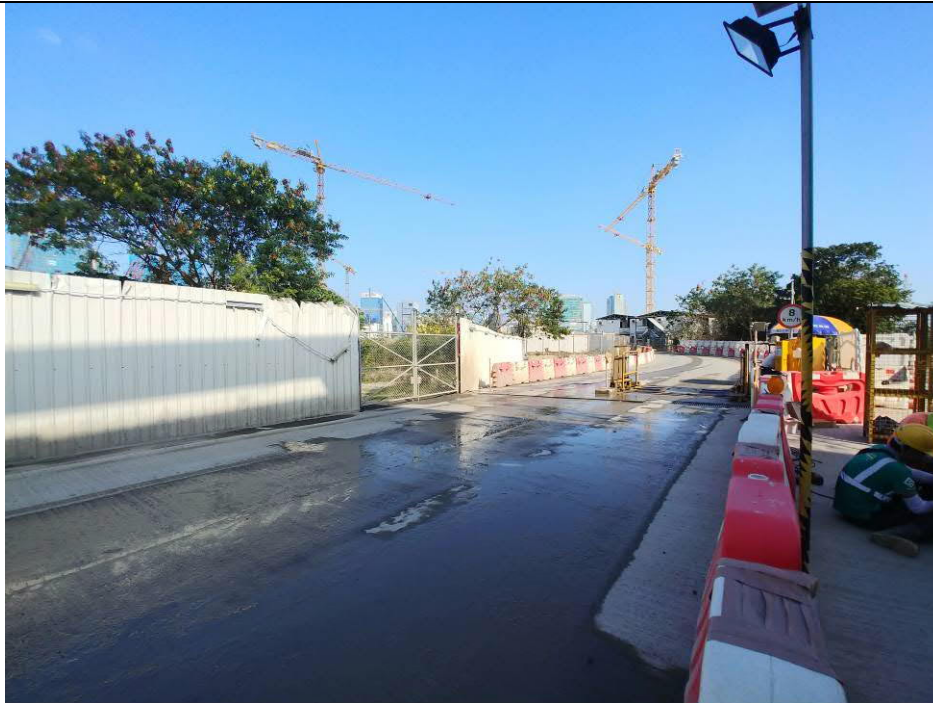
Photo 1b: Road condition at gate 3C (1 December 2020)
