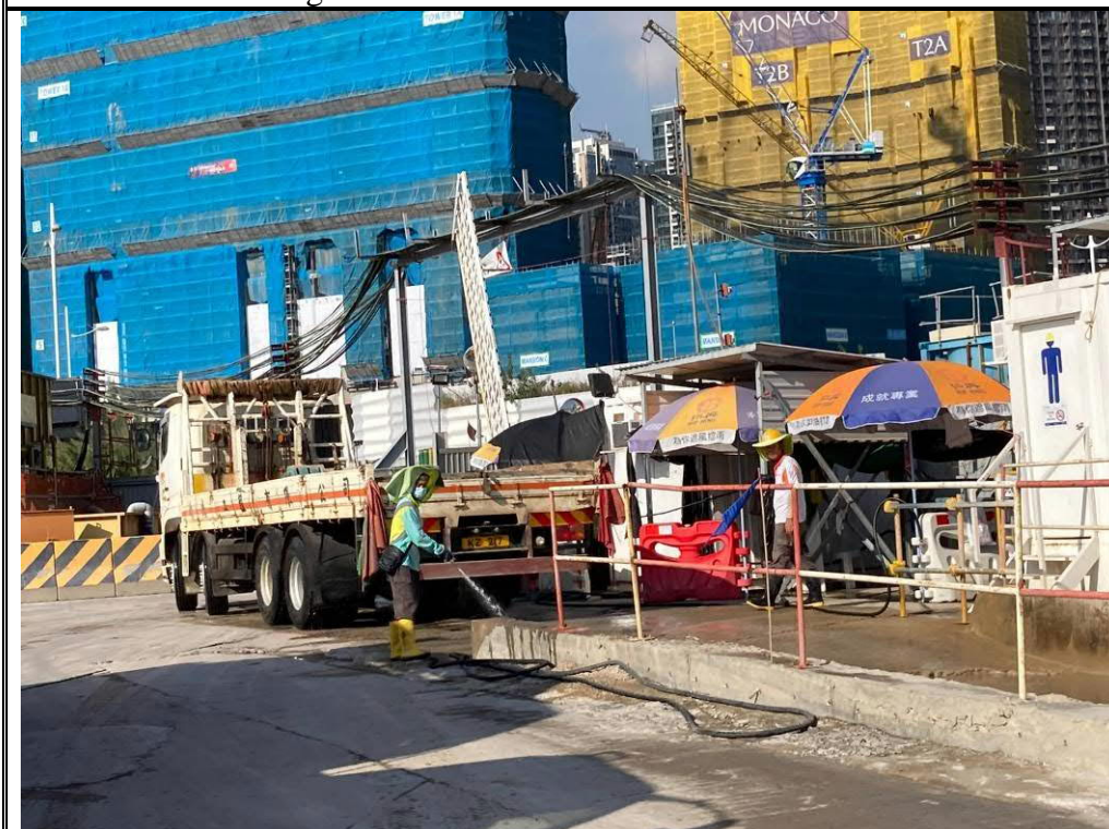
Photo 4: Workers responsible for wheel washing had been provided at all exit gates within project site
