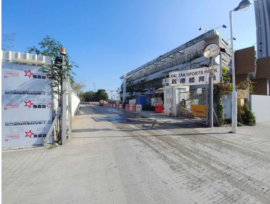
Photo 1a: Road condition at gate 3C (1 December 2020)
