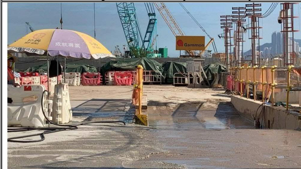
Photo 4: Workers responsible for wheel washing had been provided at all exit gates within project site.
