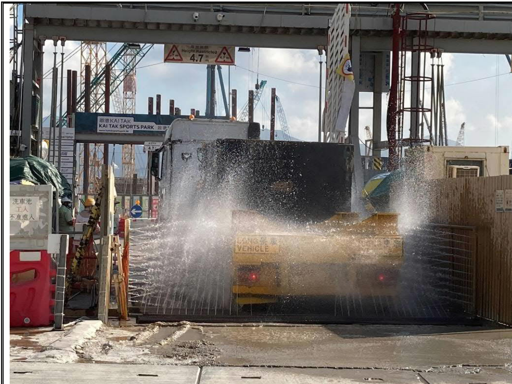
Photo 3b: Wheel washing facilities had been implemented for the passage of construction vehicles at northern gate
