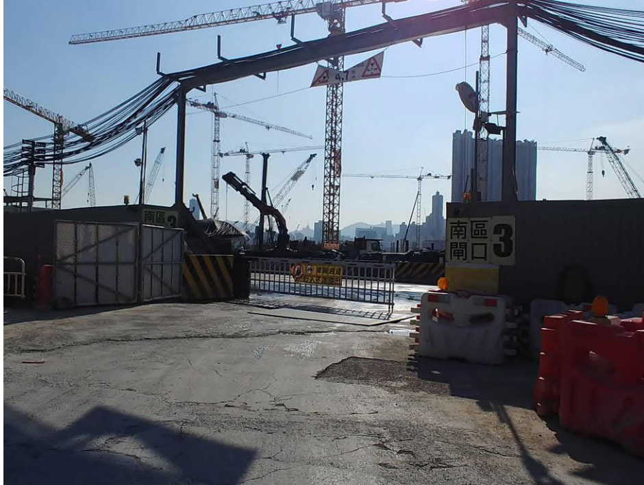
Photo 1a: Road condition at South Gate No. 3 (1 December 2020)
