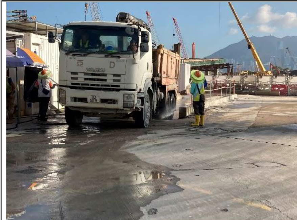
Photo 3a: Wheel washing facilities had been implemented for the passage of construction vehicles at southern gate
