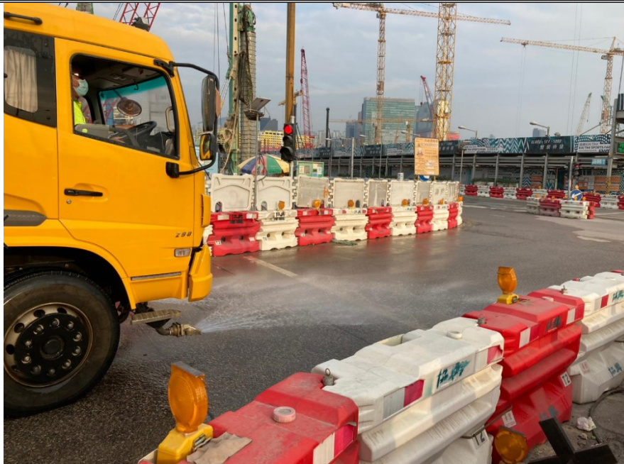
Photo 3: Water spraying truck to wash the road surface at Shing Kai Road (8 December 2020)
