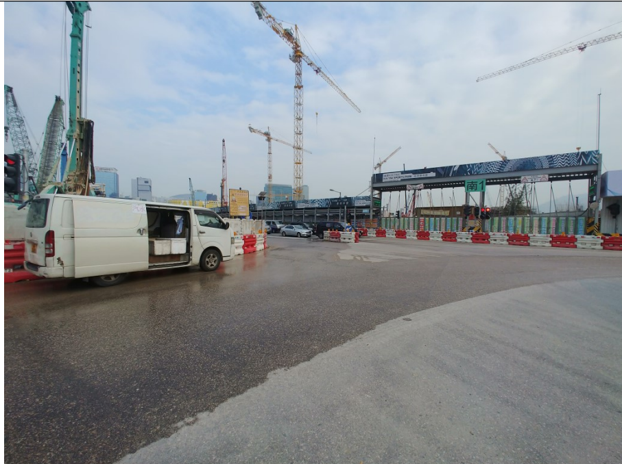
Photo 1b: Road surface condition at Gate N1 (8 December 2020)
