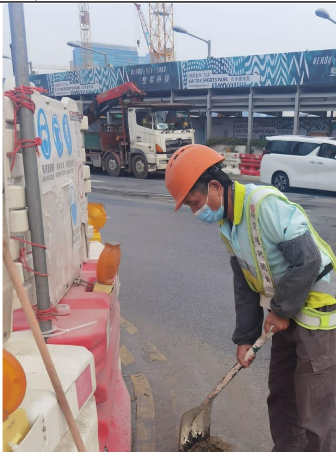
Photo 4: Worker to remove the residual sludge on road surface at Shing Kai Road(8 December 2020)
