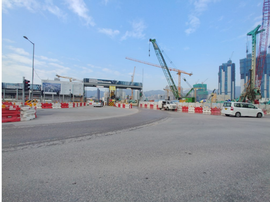
Photo 1a: Road surface condition at Gate N1 (8 December 2020)
