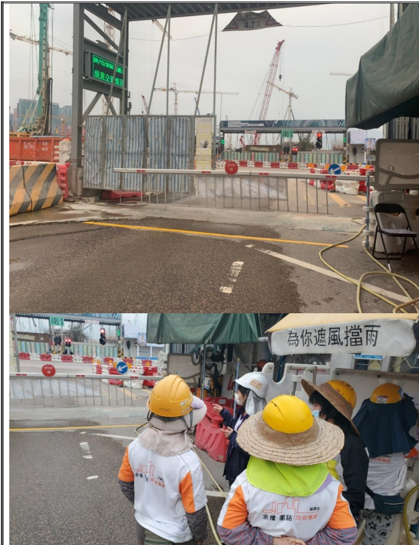
Photo 5a & 5b: Contractor set up yellow line marker at Gate N1 and instructed the workers to provide washing within the yellow line area and to prevent water jetting directing to the Shing Kai Road
