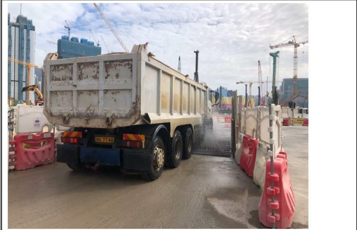
Photo 3: Wheel washing facility has been installed and implemented at all site exits.
