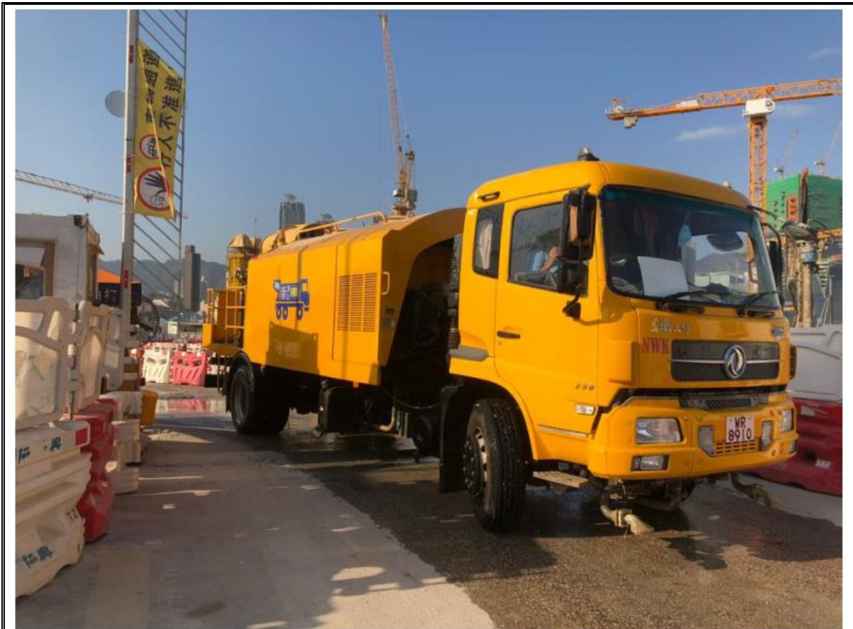
Photo 4: Water spraying by water truck has been suspended in front of North 1 Gate.
