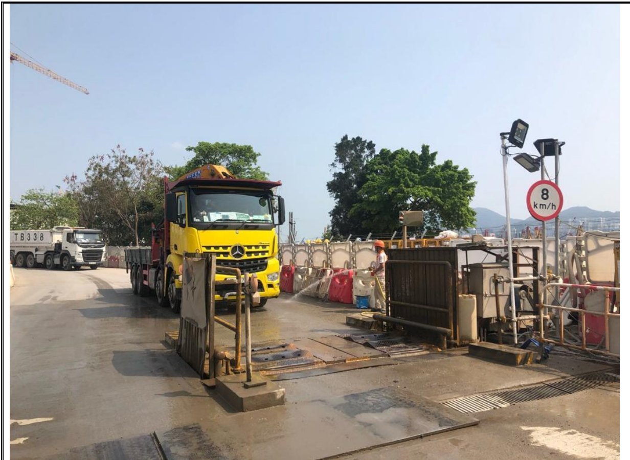
Photo 4: A worker has been assigned to maintain the tidiness at the vehicle access of the haul road 3C. (15 March 2021)
