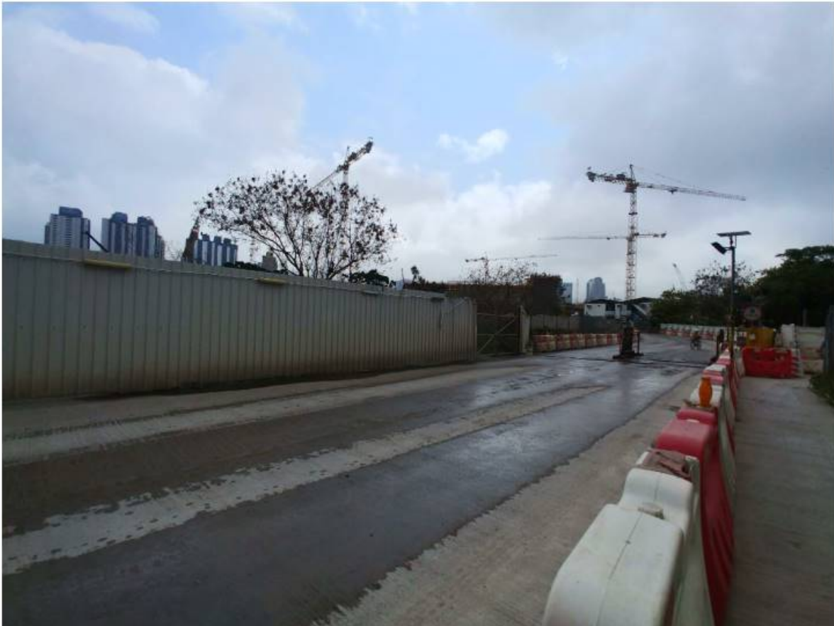
Photo 1: No dust emission at the road surface of the road 3C was observed and wet surface was maintained along the road 3C. (14 April 2021)
