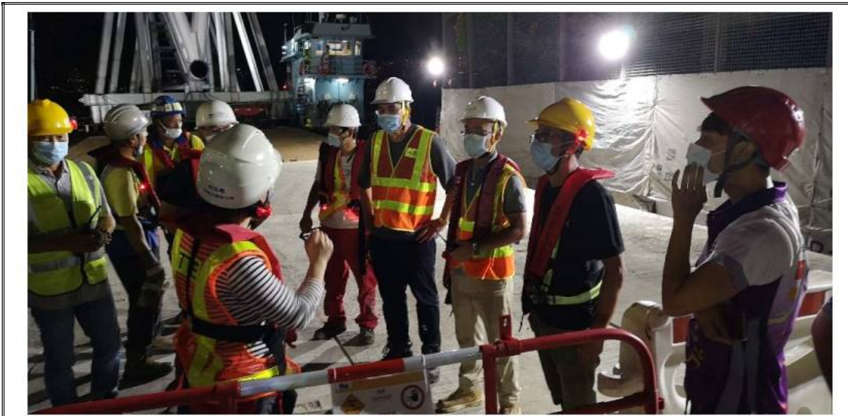
Photo 5: Pre work briefing has been provided to ensure the compliance of CNP requirement to minimise potential noise nuisance during the nighttime truss delivery.
