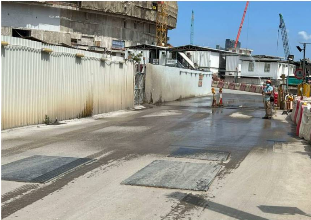
Photo 4: Worker has been arranged to maintain the road 3C surface wet. (14 April 2022)
