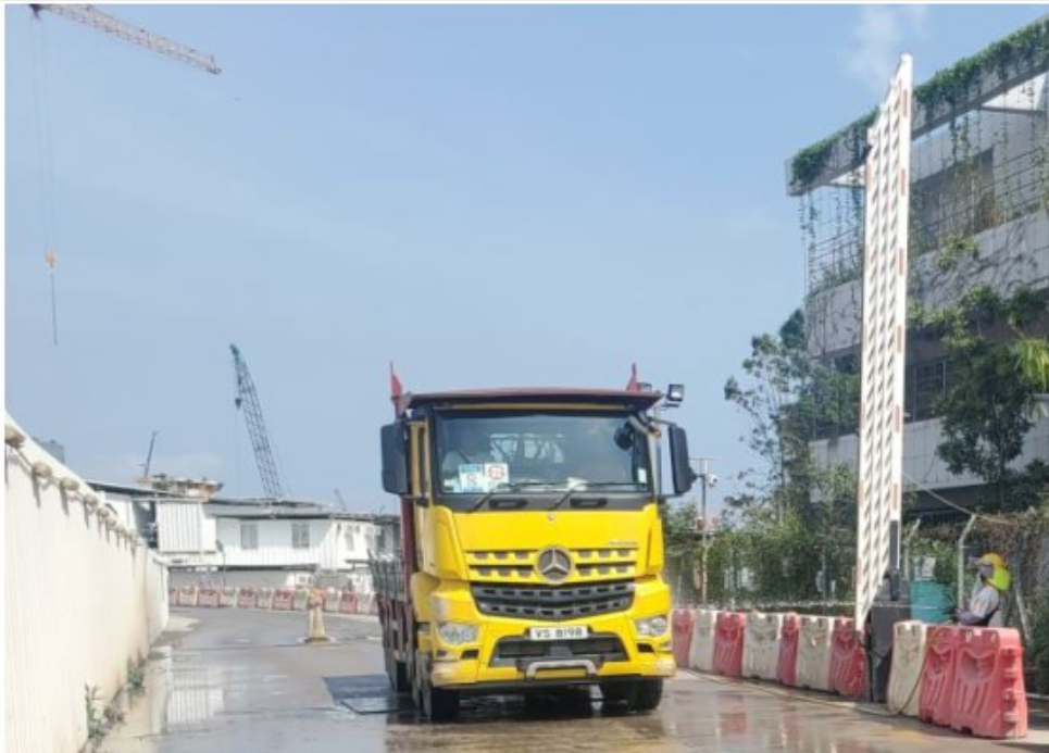
Photo 4: Worker has been arranged to maintain the tidiness at the entrance of road 3C.
