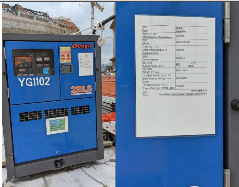
Photos 2a and 2b: Power Mechanical Equipment with Quality Power Mechanical Equipment (QPME) labels were used at site to lower the noise nuisance to the nearby residents
