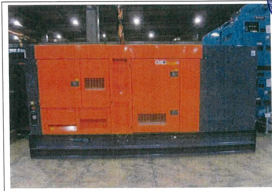
Generator, with Quality Powered Mechanical Equipment Label showing a Sound Power Level \leq 97 dB(A)
