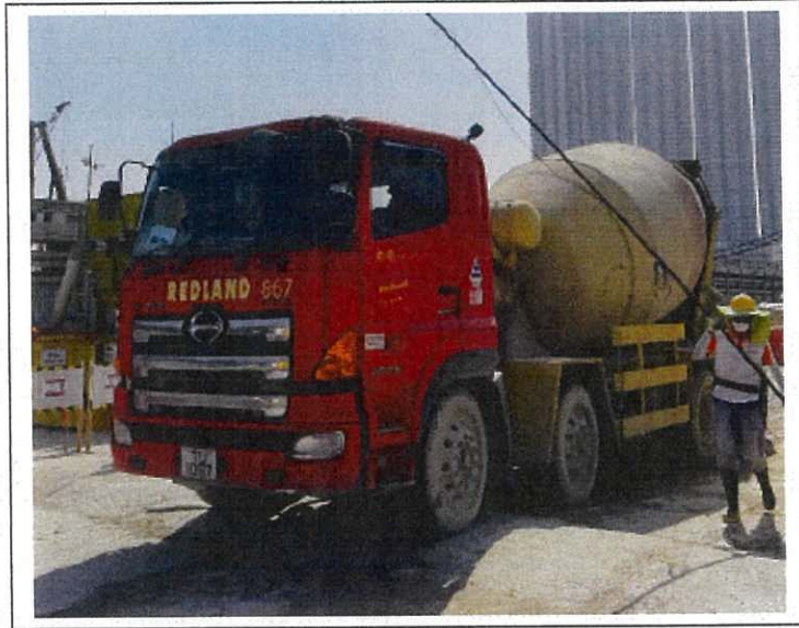
Concrete lorry mixer (Vehicle No. TU1097) 混凝土攪拌車 (車牌號碼 TU1097)
