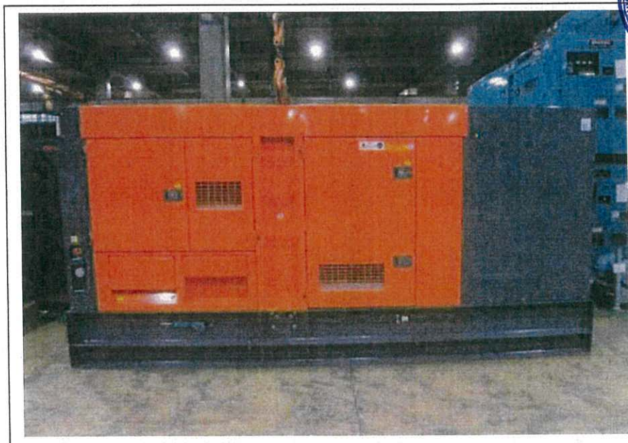
Generator, with Quality Powered Mechanical Equipment Label showing a Sound Power Level \leq 97 dB(A)
