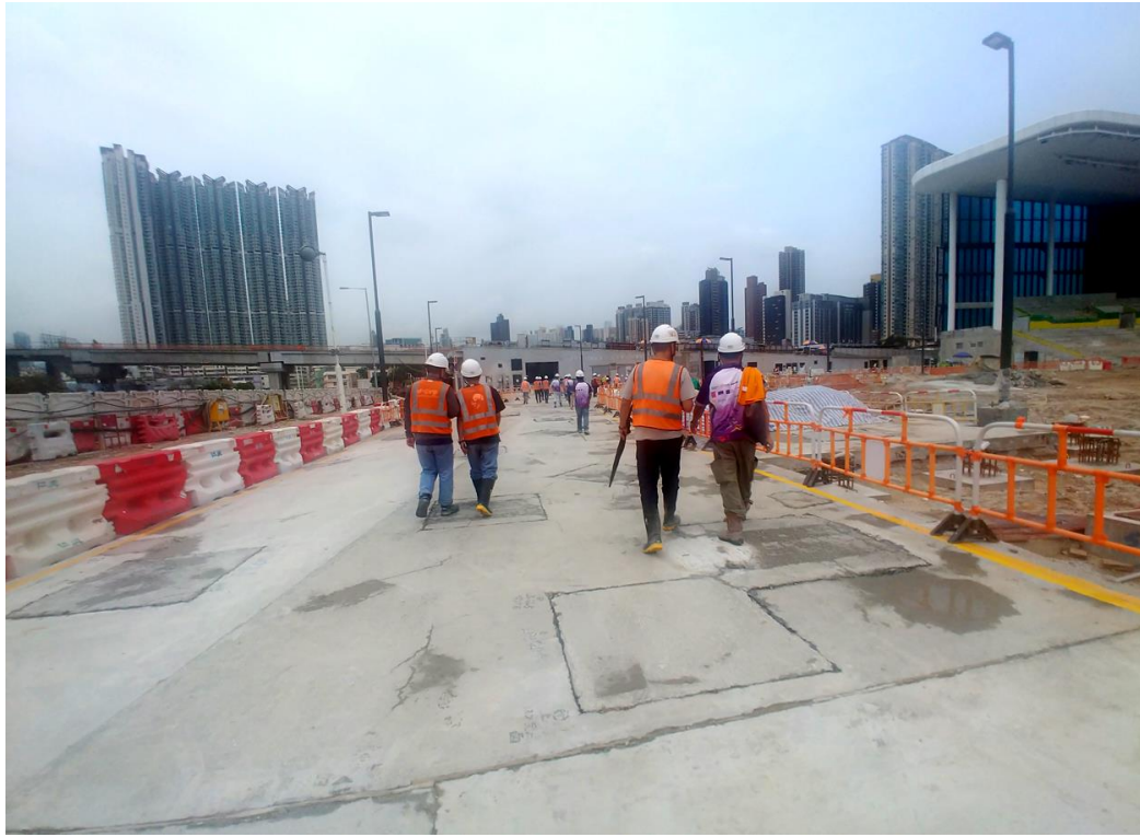
Photo 1: Photo of regular site inspection on 23 May 2023. (site area close to the Sung Wong Toi Road)
