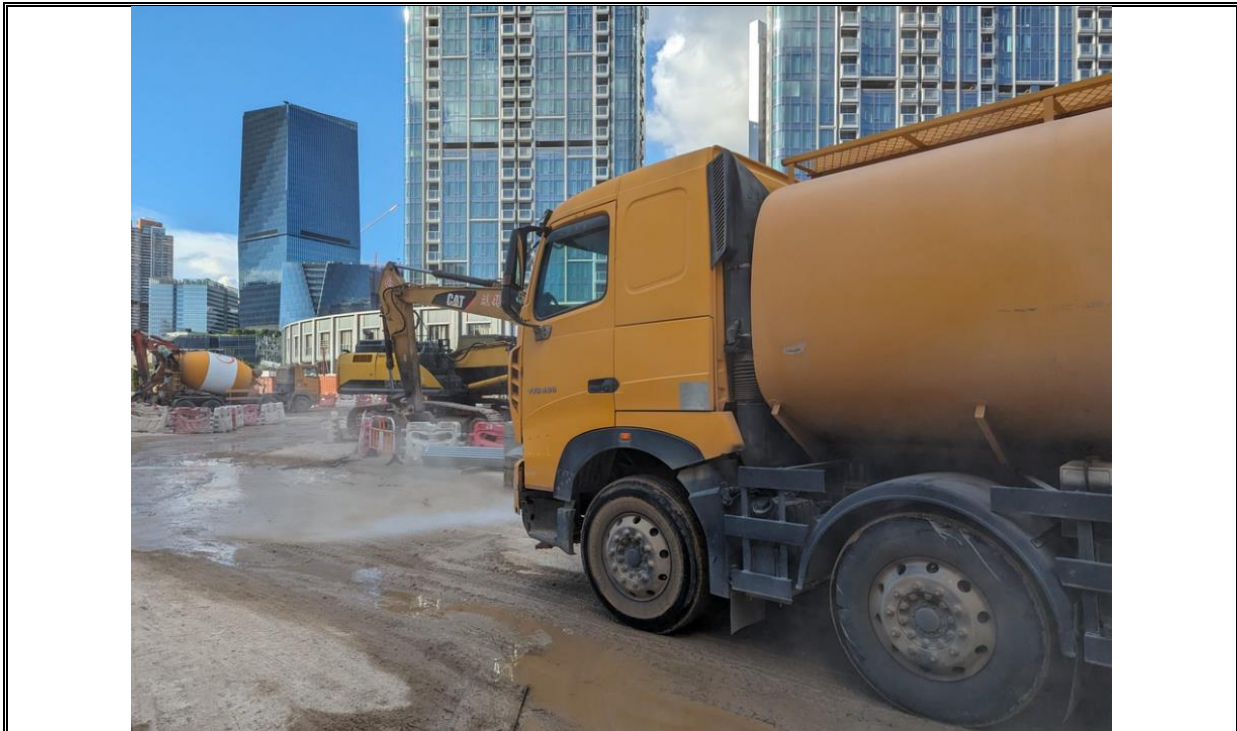
Photo 2: Water truck had been working continuously around all haul road within the site.
