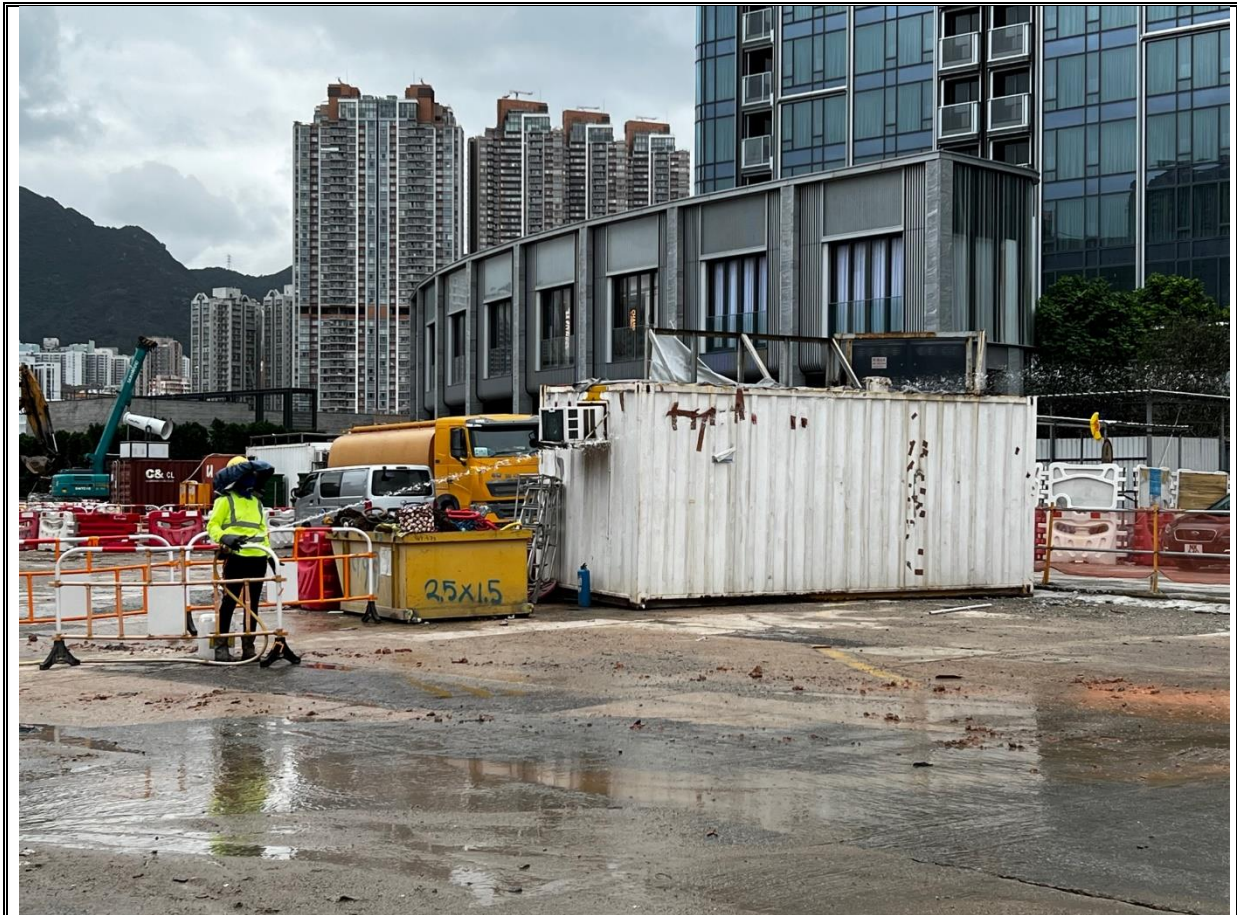
Photo 4: Water spraying was observed during regular site inspection on 19 July 2023. (site area at POS N(E))
