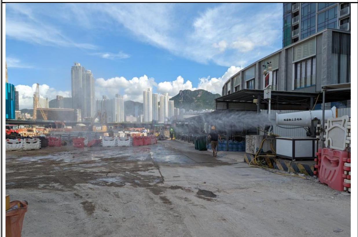
Photo 3: Water misting cannon had been installed to wet the area which water trucks cannot reach.
