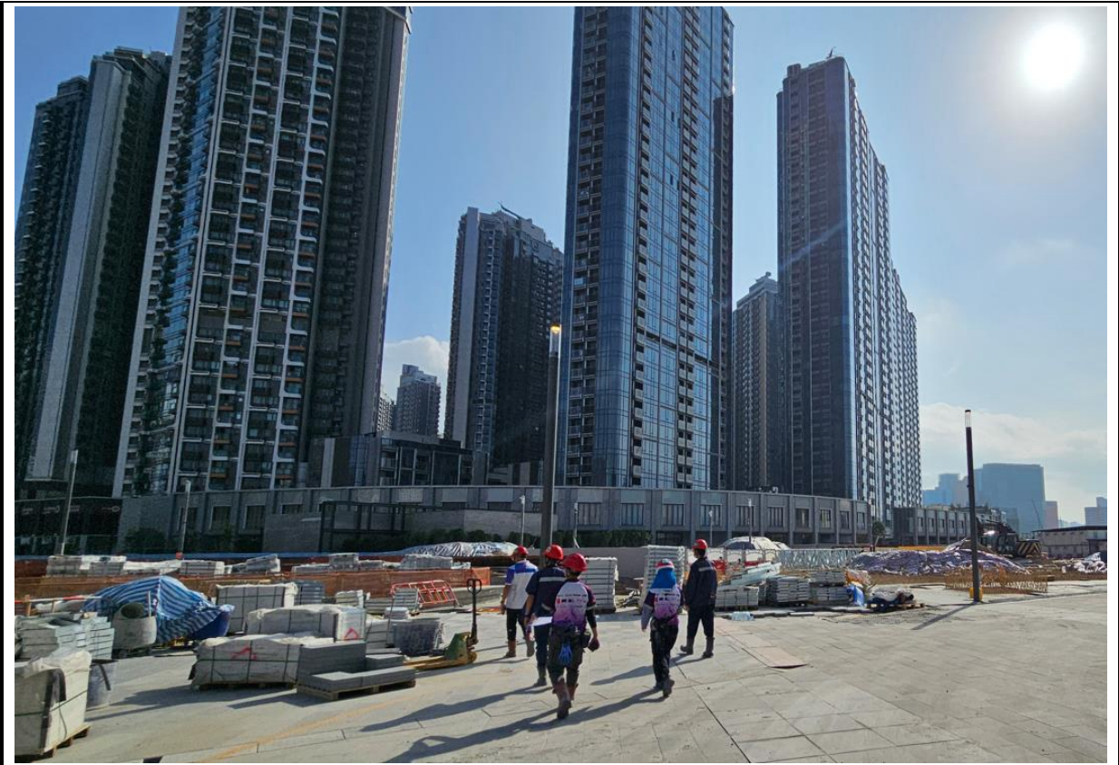
Photo 1: Regular site inspection carried out for checking covering of stockpile on site. (14 February 2024)
