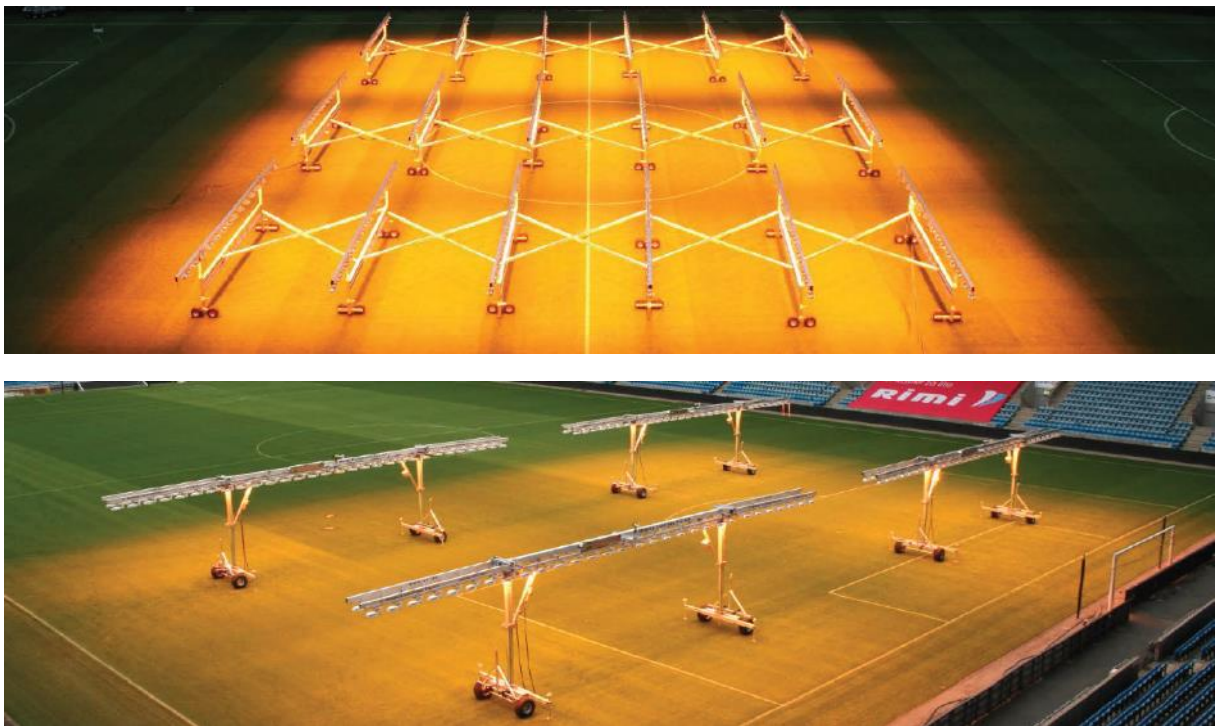
Fig. A6. Example of a lighting rig with folding arms (above) and interlocking arms (below)
