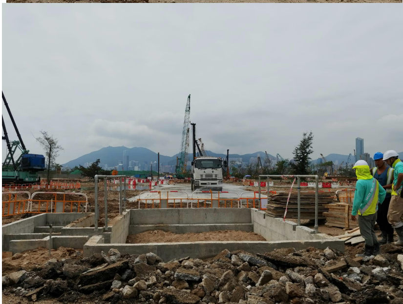
1. Water spraying has been provided on haul road in the site to minimize dust emission.
