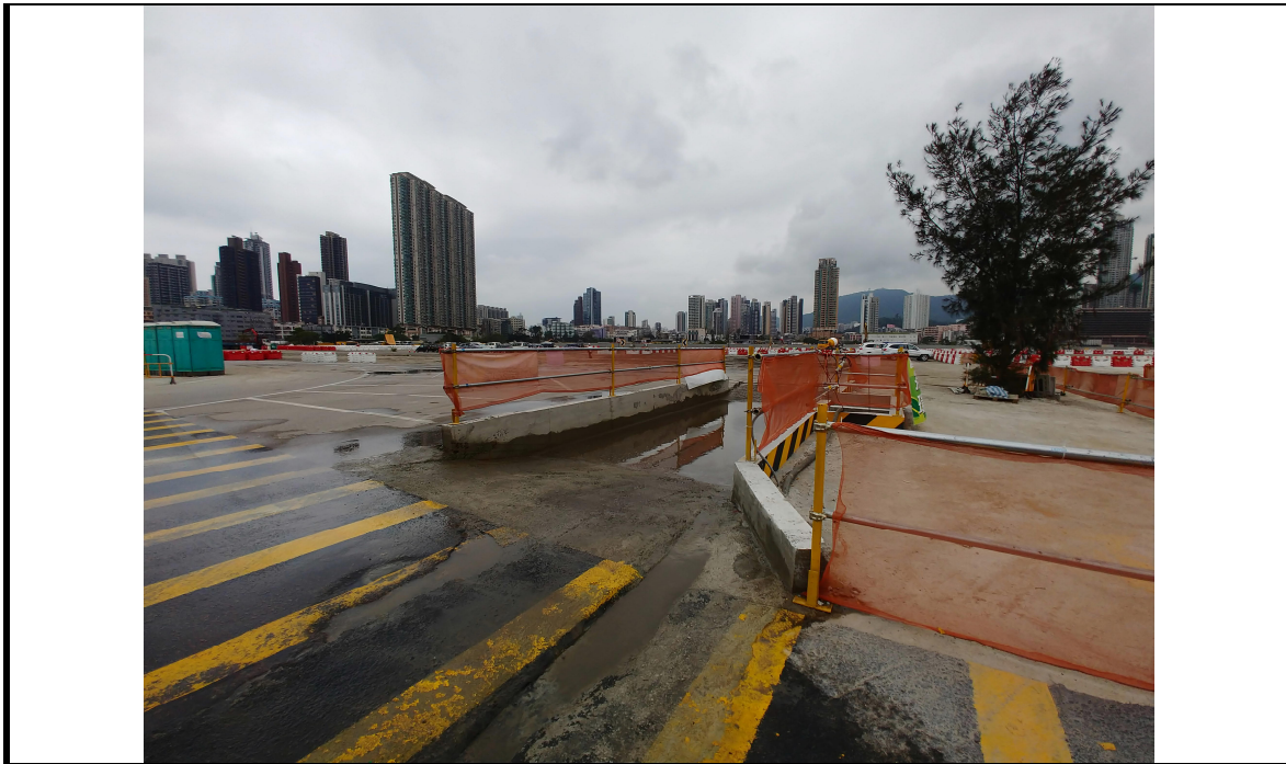
3. Wheel washing pool has been setup to minimize dust carried by leaving vehicles.
