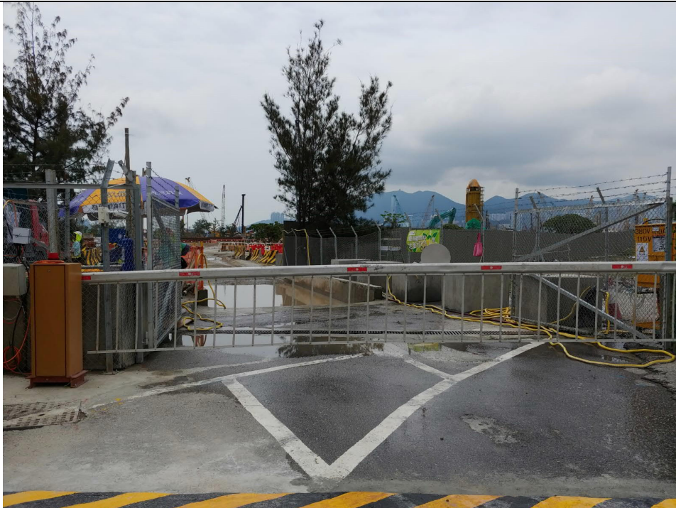
2. Wheel washing pool has been setup at the site entrance (Southern Part) to minimize dust carried by leaving vehicles.
