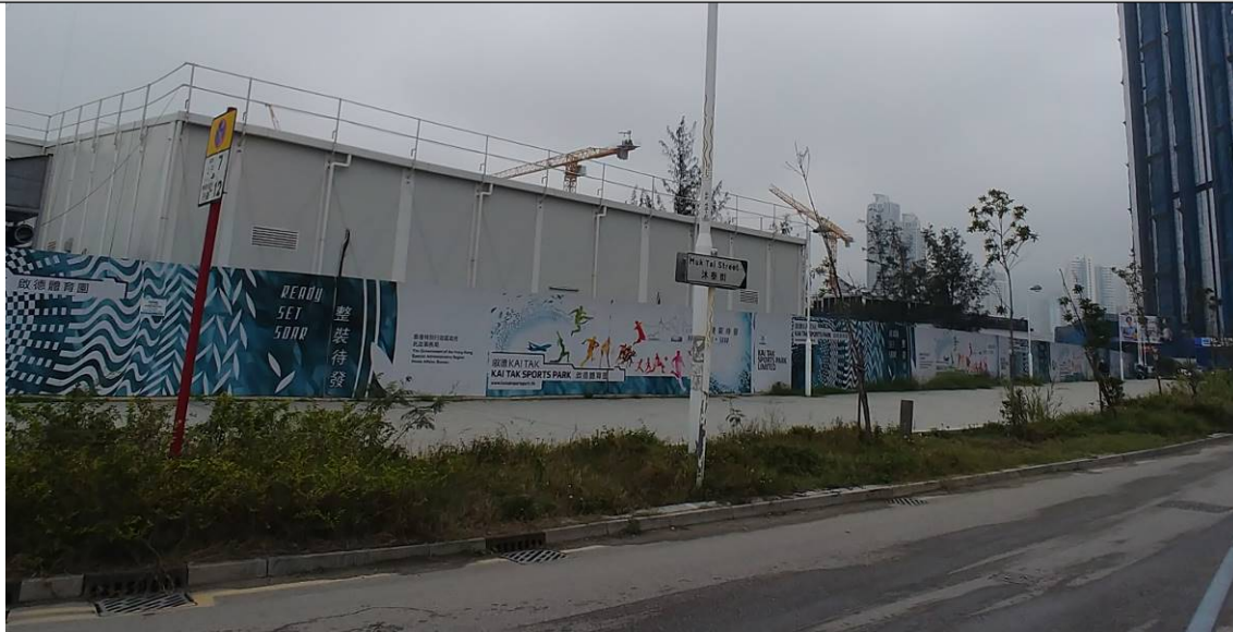
Photo 1: Site hoardings have been installed along site boundary. (Muk Tai Street direction) (5 March 2021)
