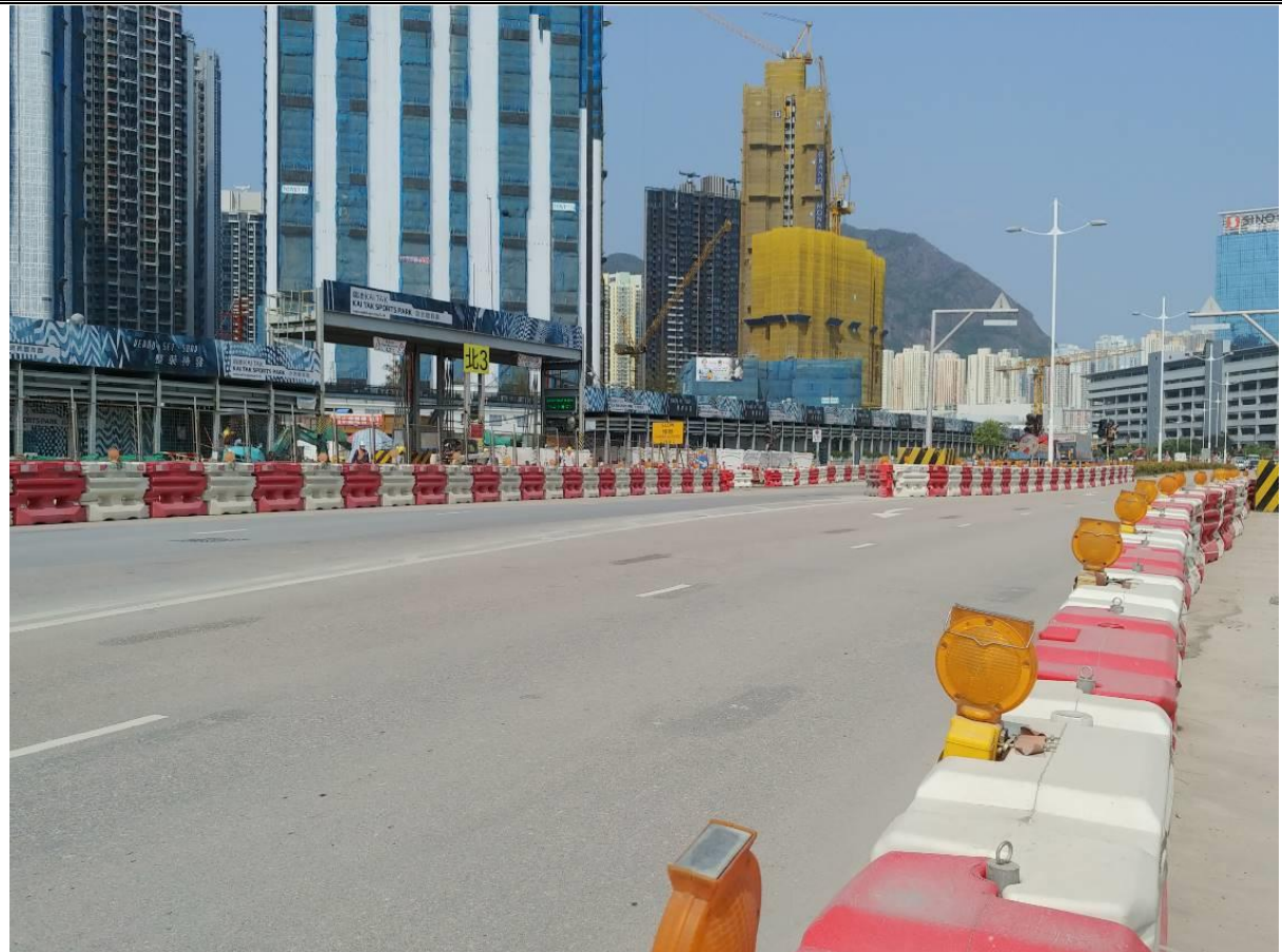
Photo 1: No discharge of muddy water was observed at vehicle entries along Shing Kai Road. (26 March 2021)
