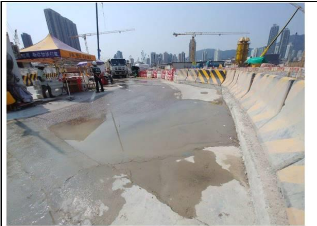
Photo 3: Earth bund was provided to trap the site runoff. (26 March 2021)
