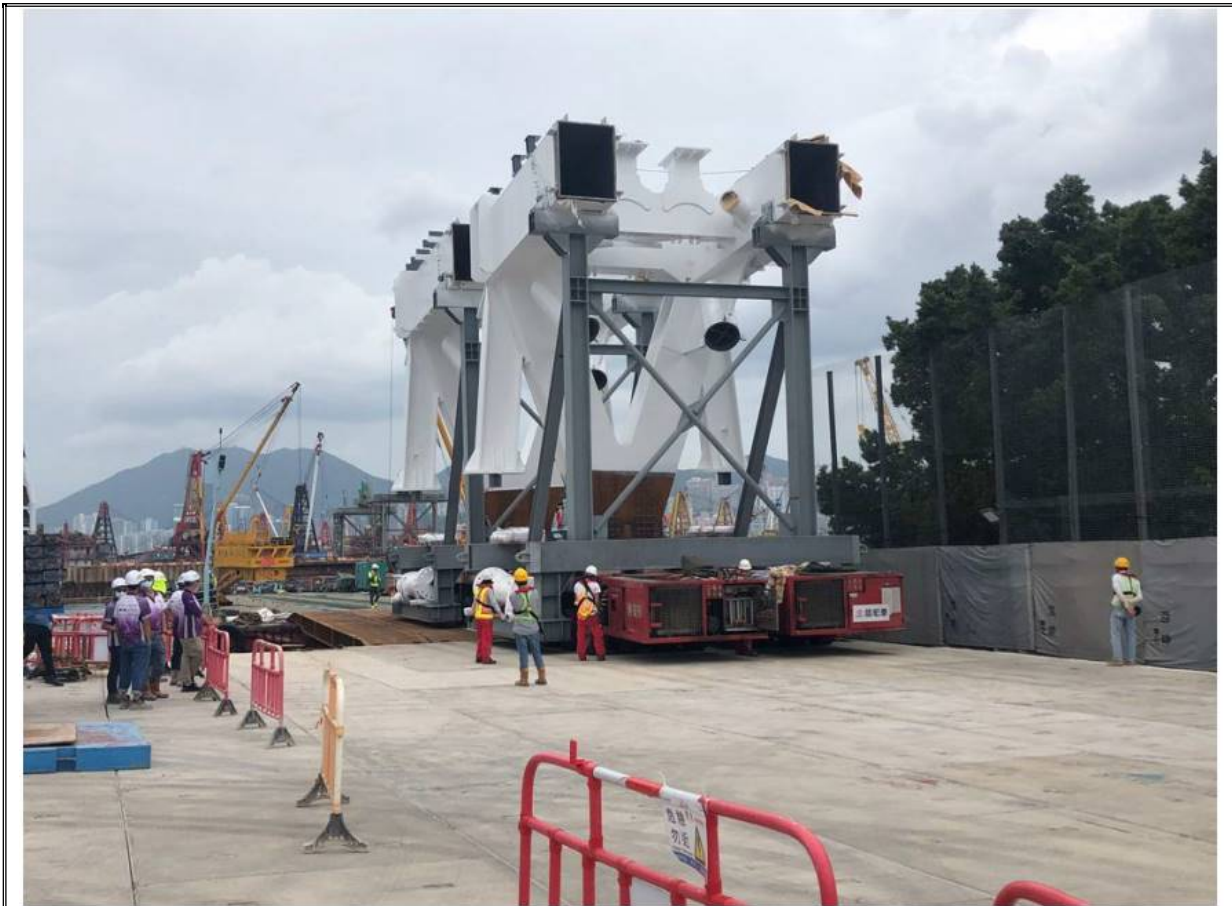
Photo 3: The truss delivery works have been scheduled in the daytime as much as practicable to minimize the noise nuisance at nighttime. (3 November 2021)
