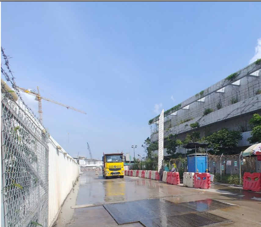
Photo 2: No soil and sand was observed on the road surface of nearby pavement on 29 April 2022.
