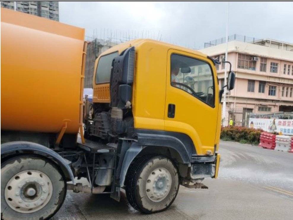
Photo 3: Water truck has been provided regularly at road 3C and entrance for dust suppression.
