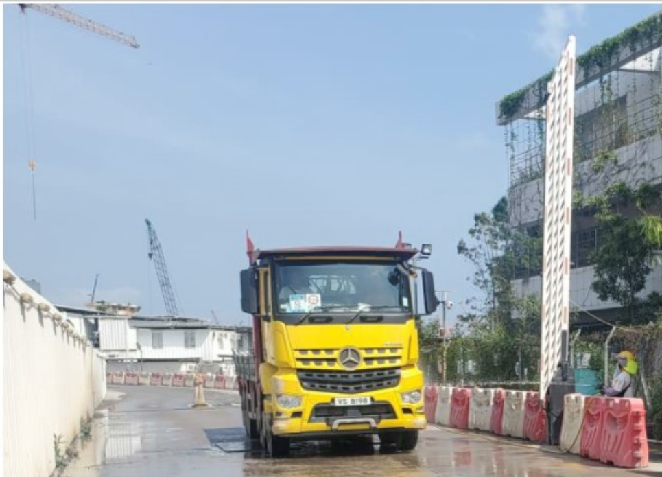
Photo 4: Worker has been arranged to maintain the tidiness at the entrance of road 3C.
