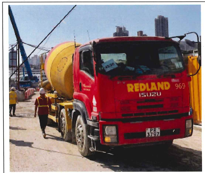
Concrete lorry mixer (Vehicle No. PR3797) 混凝土攪拌車 (車牌號碼 PR3797)
