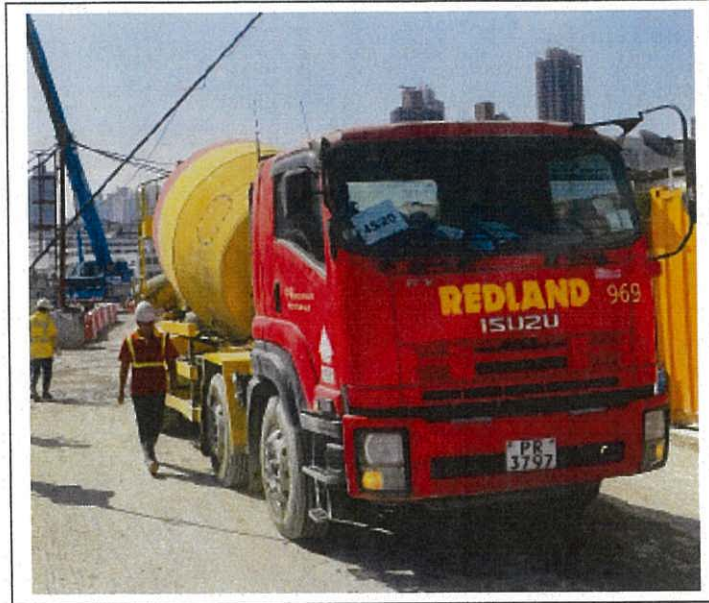
Concrete lorry mixer (Vehicle No. PR3797) 混凝土攪拌車 (車牌號碼 PR3797)
