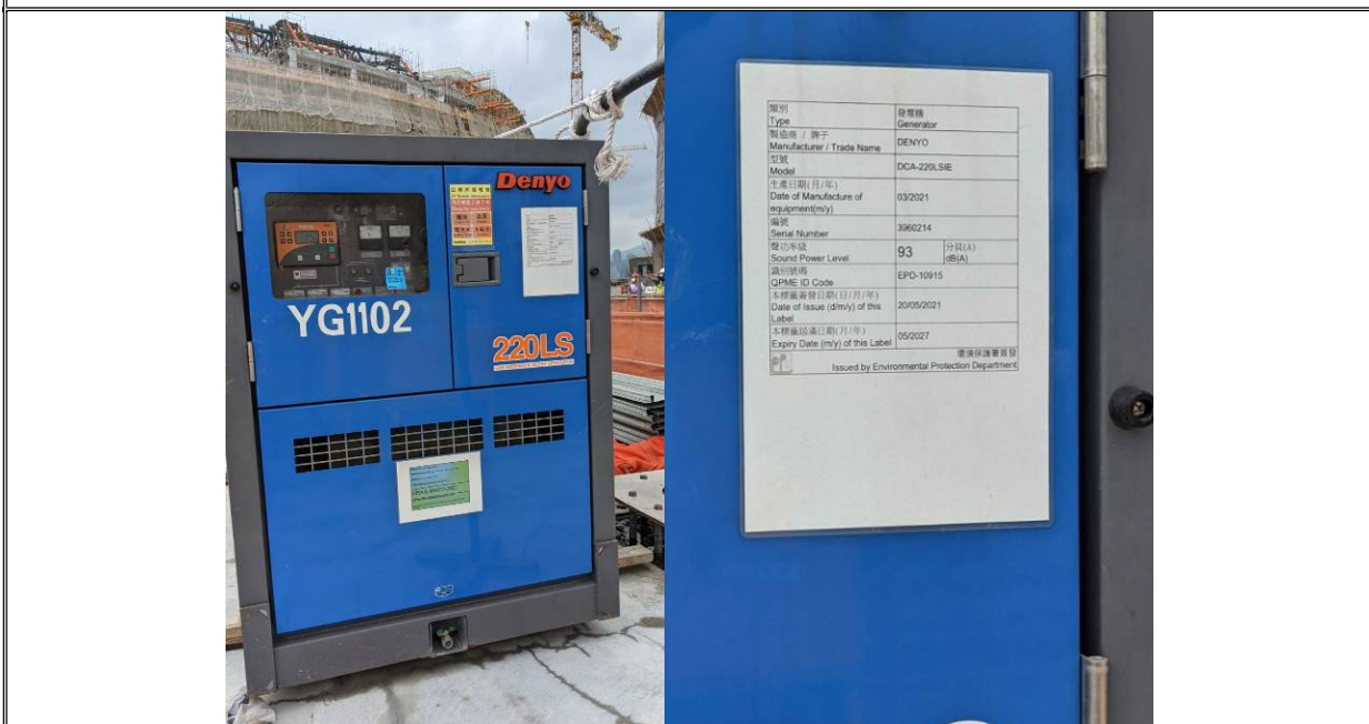
Photos 2a and 2b: Power Mechanical Equipment with Quality Power Mechanical Equipment (QPME) labels were used at site to lower the noise nuisance to the nearby residents
