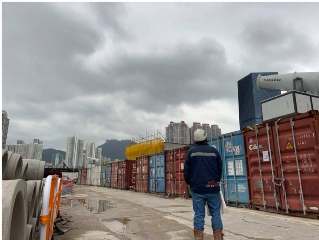
Photo 3: Site staff will be arranged for daily checking to ensure no operation of mist cannon by end of working day.
