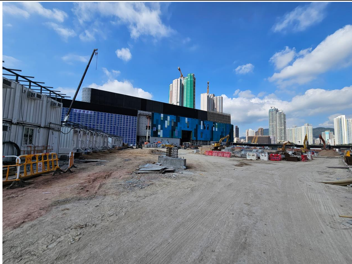
Photo 1: Photo of site inspection on 3 November 2023. (site area close to the Muk Tak Street)
