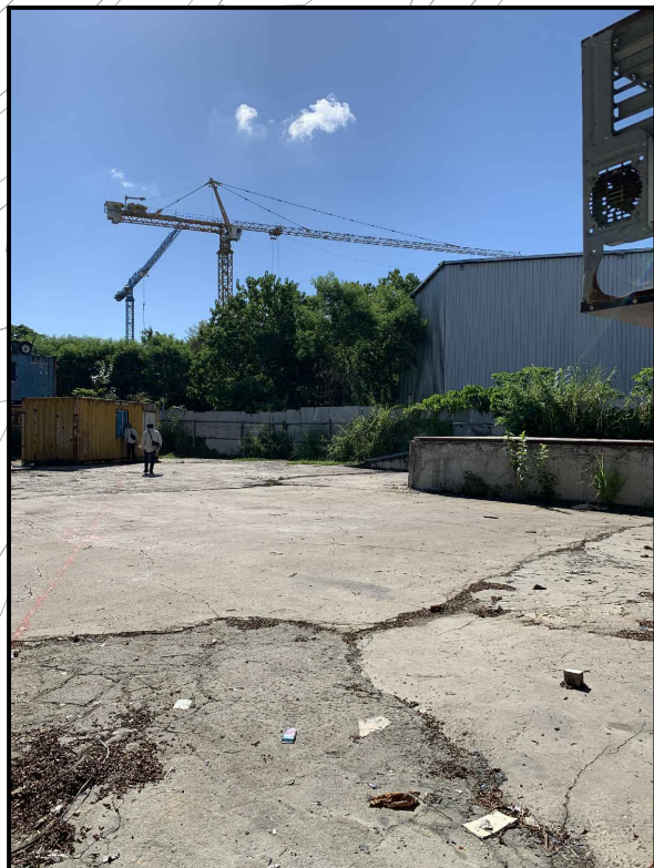
6_Cracks on superficial layer of ground
