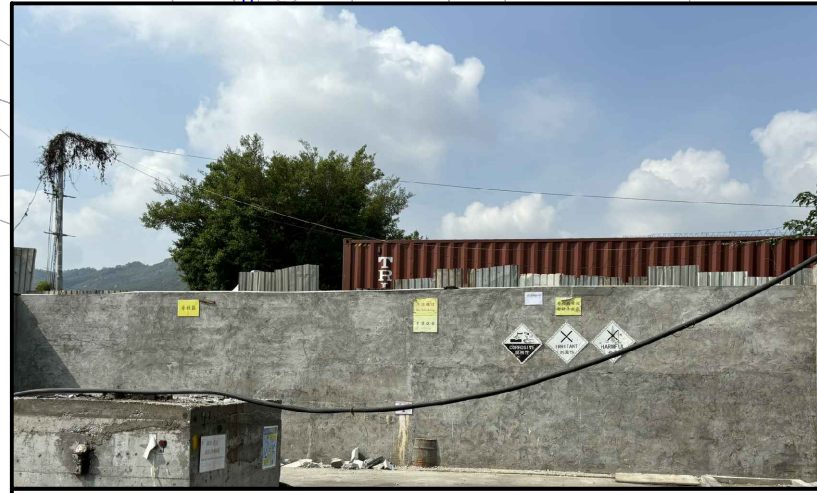
2_Storage areas including a chemical storage area (waste batteries) on fully paved ground at E136
