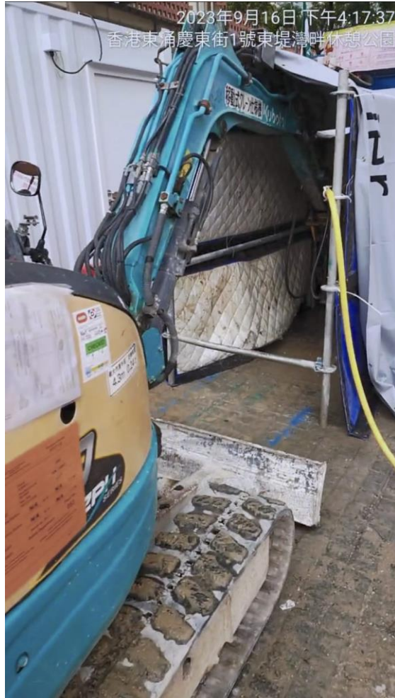
Photo E2.5: Sample Photo of Semi Noise Enclosure Screening the Breaker Head of Mini-robot Mounted Breaker
