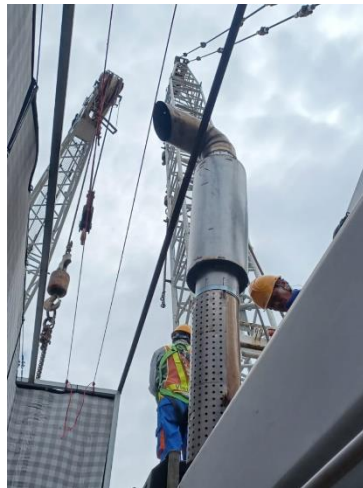
Photo E5.2: Sample Photo of Silencer at Exhaust
