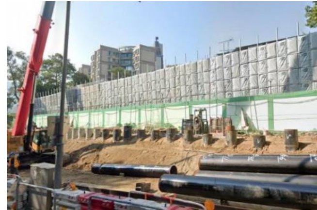
Photo E2.3: Sample Photo of Noise Barrier along Site boundary
