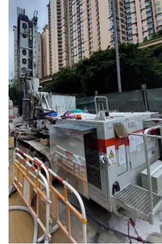
Photo E5.3: Sample Photo of Acoustic Plenum
