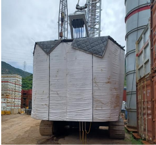
Photo E5.1: Sample Photo of Barriers at Engine Box
