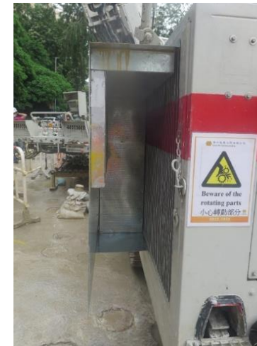
Photo E5.4: Sample Photo of Acoustic Plenum
