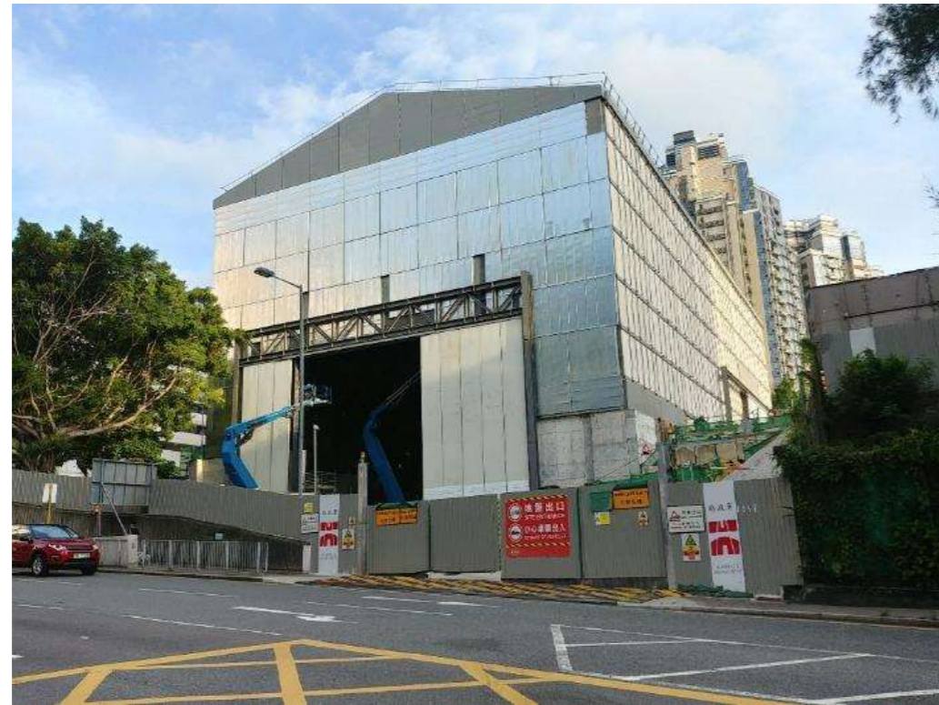
Photo B1.1: Sample Photo of Noise Enclosure (Central Kowloon Route – Centre Tunnel)
