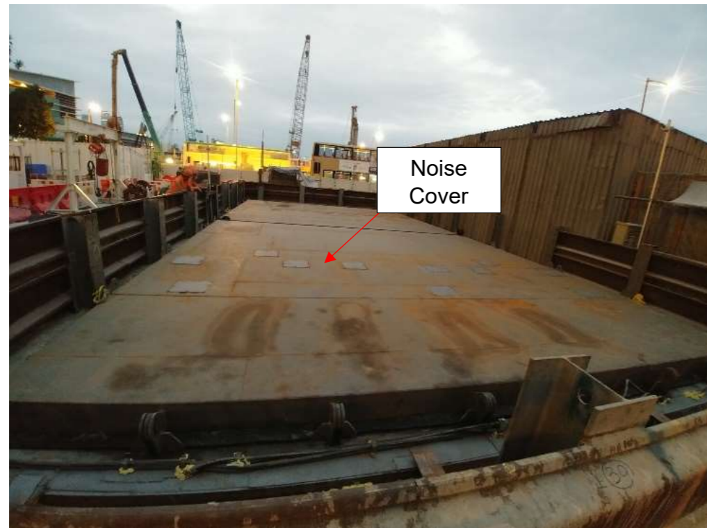
Photo B1.2: Sample Photo of Noise Cover (Central Kowloon Route – Centre Tunnel)
