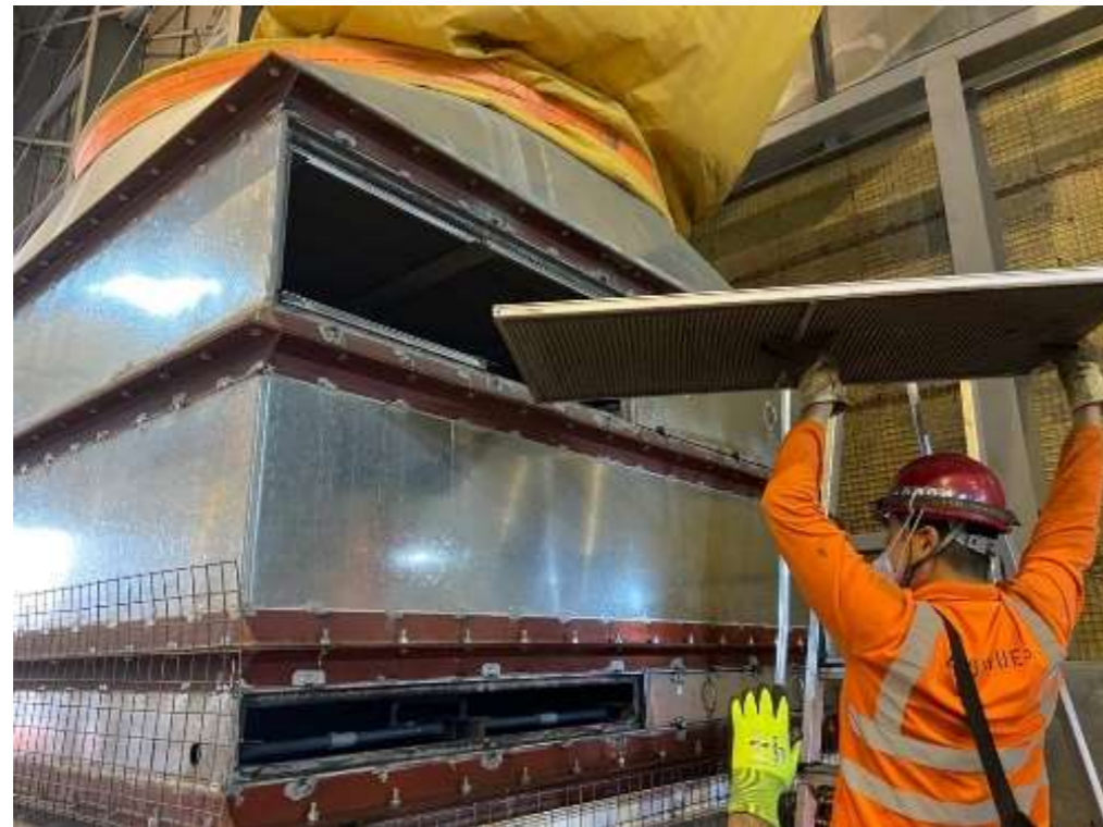
Photo C1.2: Sample photo of Exhaust duct with Dust Filter and Mist Nozzle
