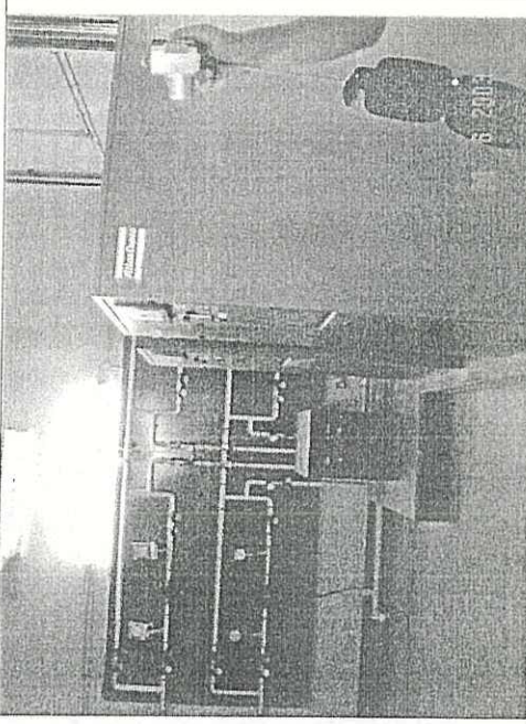
Photo 2.21: Air compressor room
