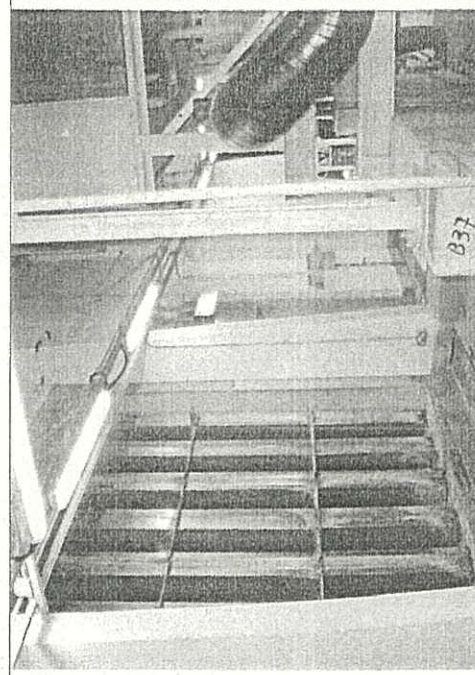
Photo 5.98: Acoustic Louvers installed in SIH Chiller Plant Room
