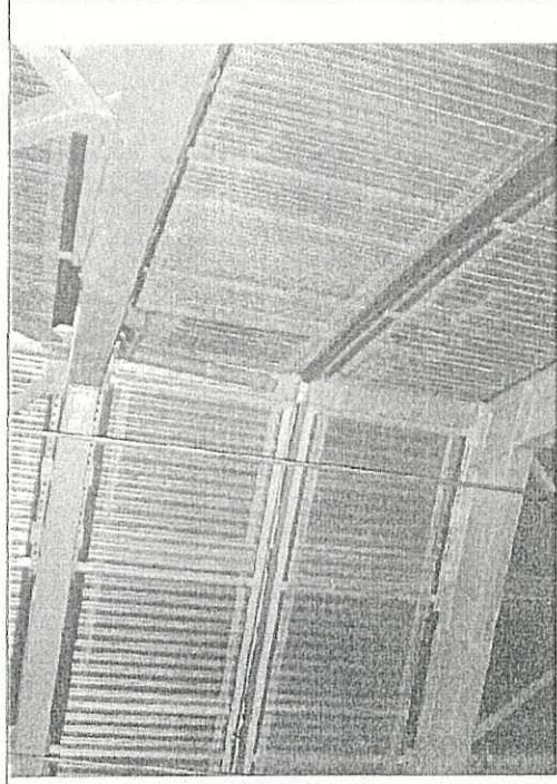
Photo 5.21: Gap Identified Inside Enclosure (Roof)
