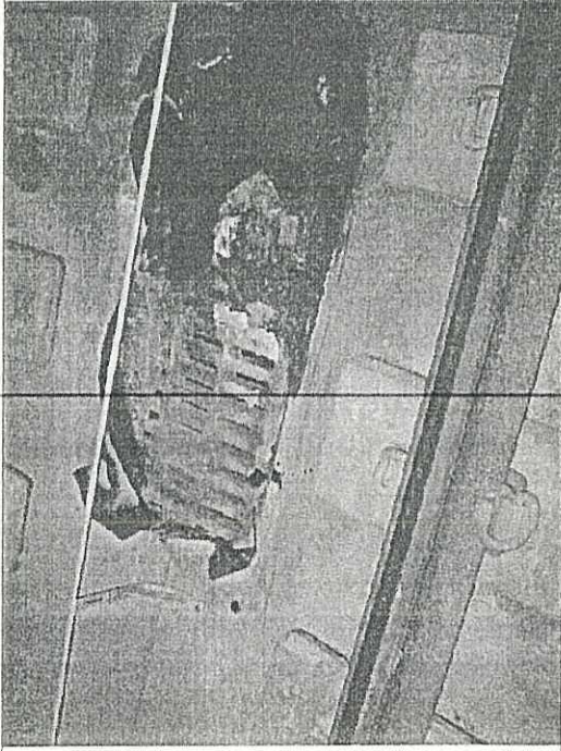
Photo 3.40: Silt trap in Kwai Tsing Tunnel
