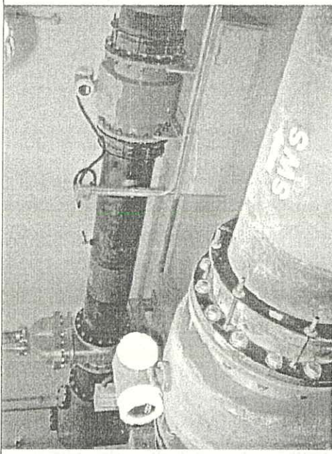
Figure 3.16 Cooling Water Plant Room
