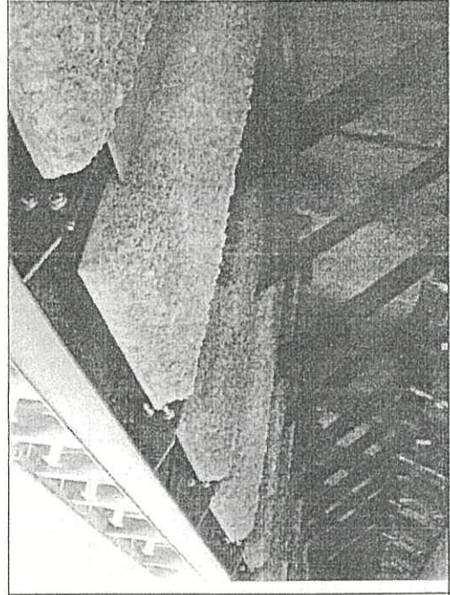
Photo 5.67c Acoustic panel at trackside walkway
