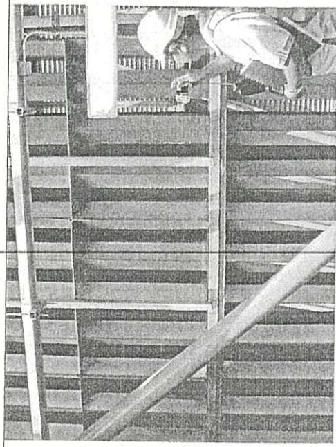
Photo 2.4: Silencers for the Chiller Plant
