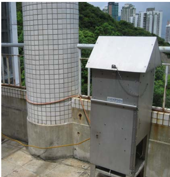
Air Quality Monitoring Station (AM1)
