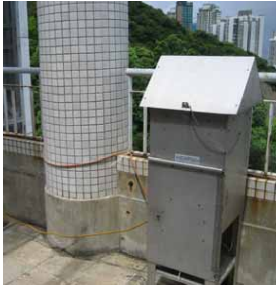
Air Quality Monitoring Station (AM1)
