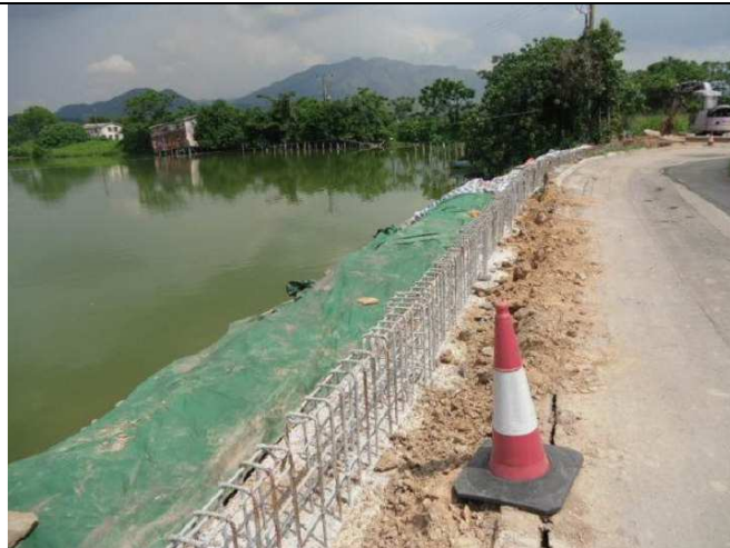
Photo (vii) – The slope area next to the fish pond was covered with tarpaulin to prevent the generation of muddy water during rainstorm.
