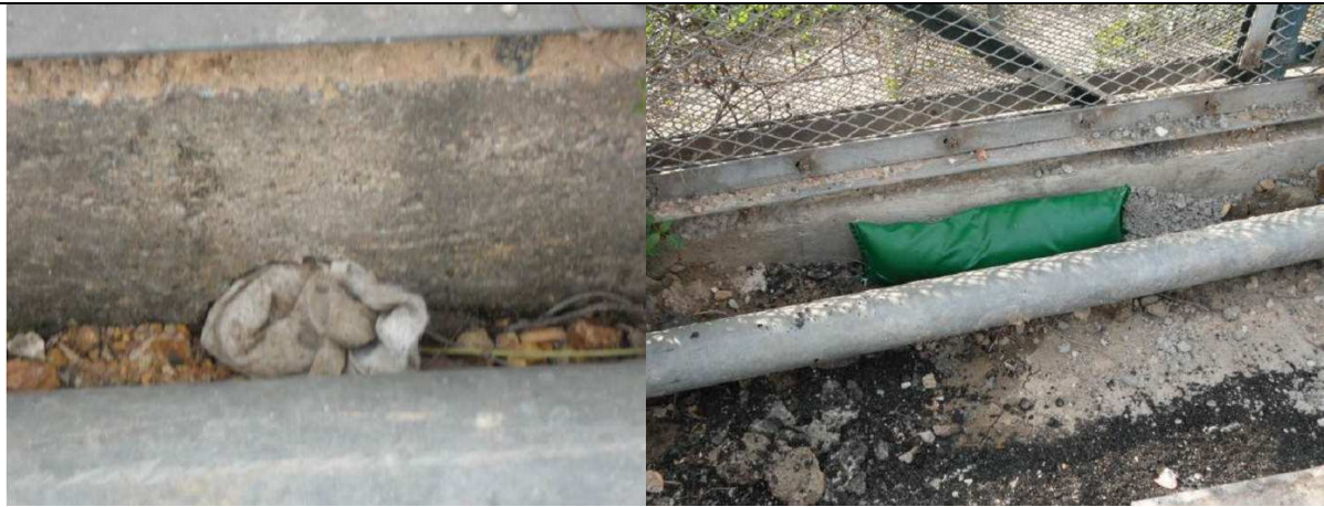
Photo (iv, v) – The hole at the bottom of the Primary Boundary Fence was filled with geotextile and covered with sand bag to prevent the run-off spillage.
