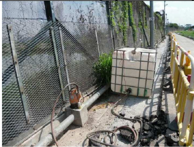
Photo (vi) – Stand-by water pump was provided by the Contractor to collect the wastewater to sedimentation tank.
