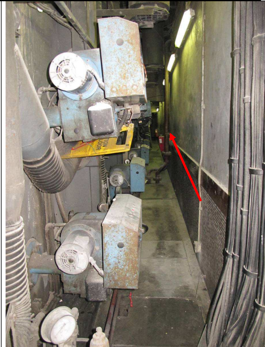
Description: External Main Fuel Pipe to Cremator (CR1)
