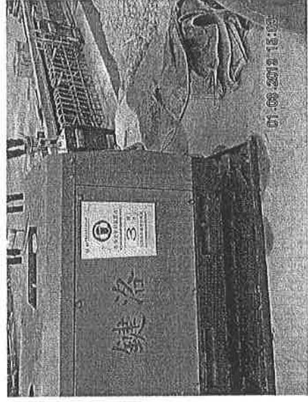
Photo 130301_005 -- Leakage of oil was noticed from a generator without drip-tray near Gate No. 70.
