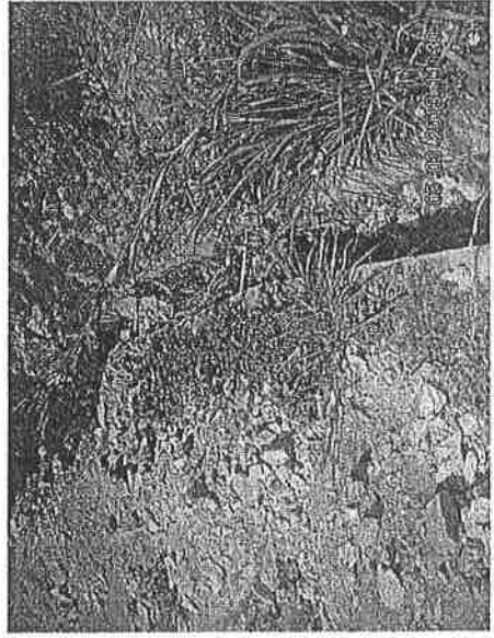
Photo 130306_002 – Gravel and mud were still noticed at U-channel near 121 fencing.
