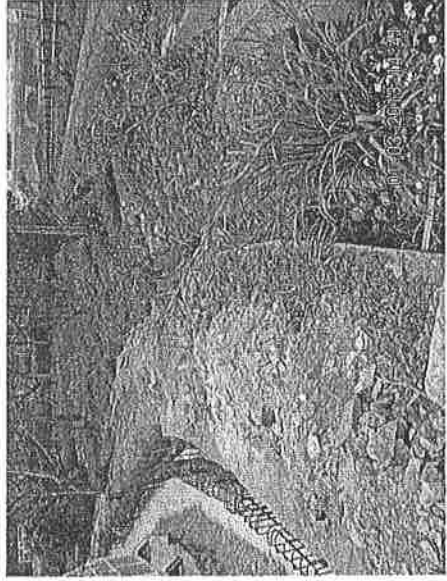
Photo 130301_002 -- Gravel and mud were noticed at U-channel near 121 fencing.
