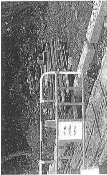
Photo 130515_001 – C&D waste observed at Man Kam Road site was improved.
