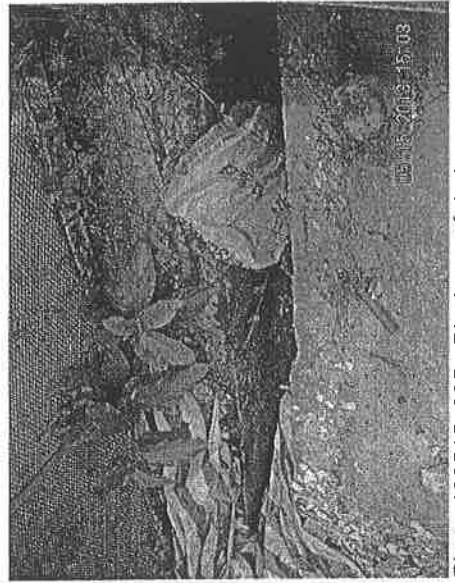
Photo 130515_005 - Blockage of drainage was observed near fence 121 at Lo Wu site.
