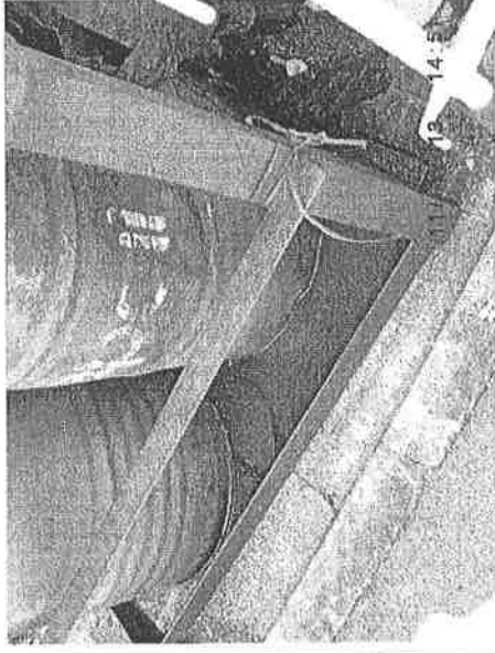
Photo 130911_005 – A drip tray with standing rain water was observed near Fence 135 at Man Kam Road site.
