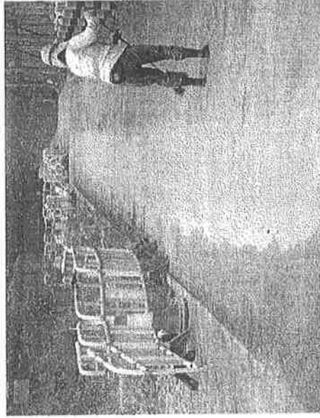
Photo 131219_001 – Mud trail on the access road observed near Fence No. 141 in Man Kam To site was improved.
