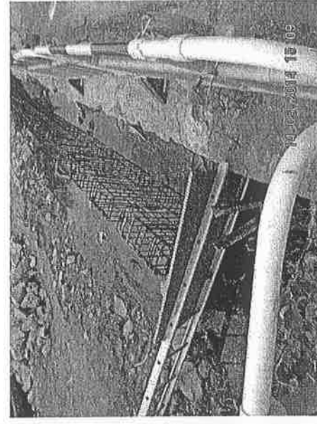
Photo 140514_006 – Stagnant water pond was observed near Gate No. 47 in Pak Fu Shan site.
