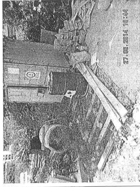
Photo 140627_004 - Oil tank without drip tray was observed in New Road site.
