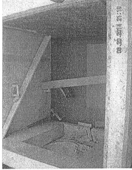
Photo 140620_003 – Stagnant water was observed near the middle section of New Road site
