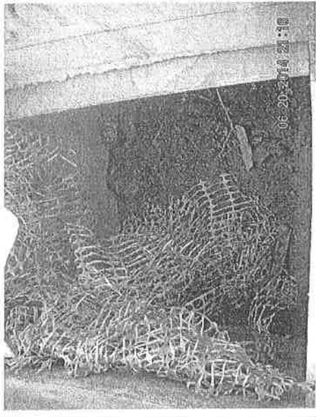
Photo 140620_001 – Stagnant water observed near the middle section of New Road site was removed.
