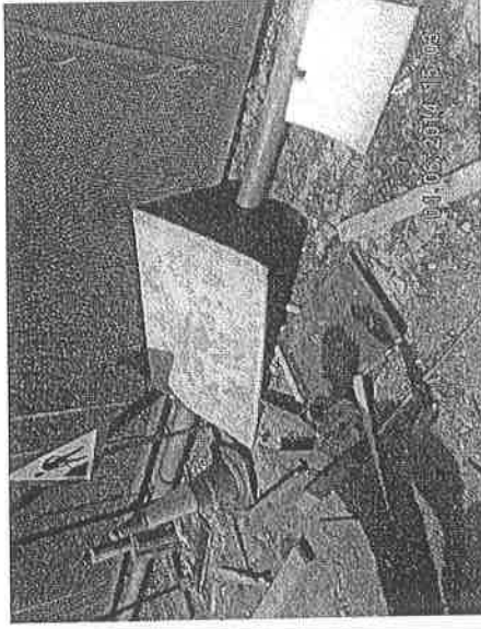
Photo 140604_003 – Rubbish was observed near Gate No. 68 in Lo Wu site.
