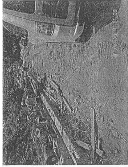
Photo 140709_004 – Dusty road surface was observed in New Road site.
