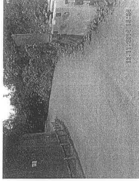
Photo 141112_003 – Dusty materials was observed at the entrance of New Road site.
