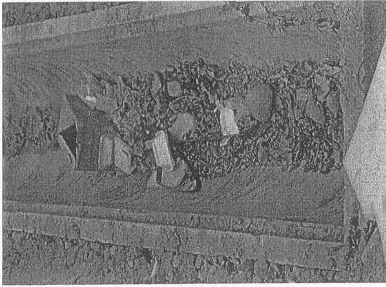
Photo 150211_001 – General refuse was observed near the end section of New Road site.
