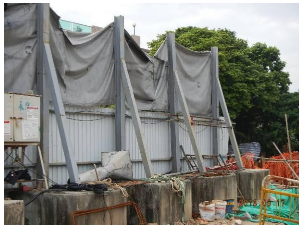
Fig. 2 –The noise barriers were provided for sheet piling activities to minimize the noise impact.
