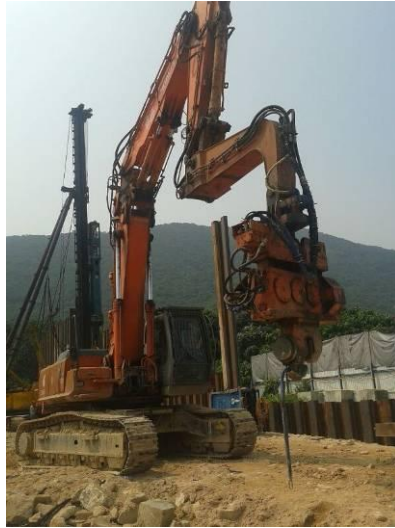
Fig.1 – sheet piling activity was wrapped up with plastic material to minimize noise generation.
