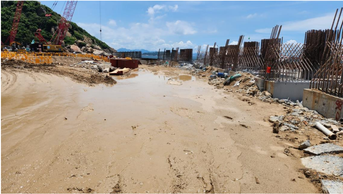
Figure 4: Site Photo of Main Haul Road Taken during Site Inspection on 12 June 2023
