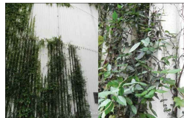
VERTICAL GREENERY REFERENCE IMAGE OF Trachelospermum jasminoides IN SHA TIN SEWAGE TREATMENT PLANT
