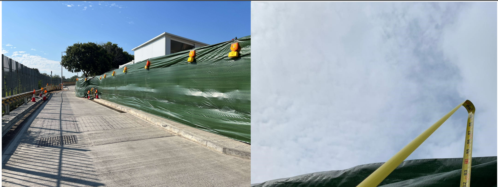
The site barrier fence next to Shek Sheung River (Sidestream) is completed
