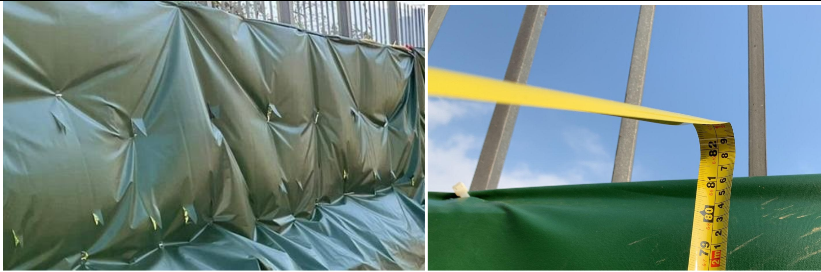
The site barrier fence next to Shek Sheung River (Area C) is completed
