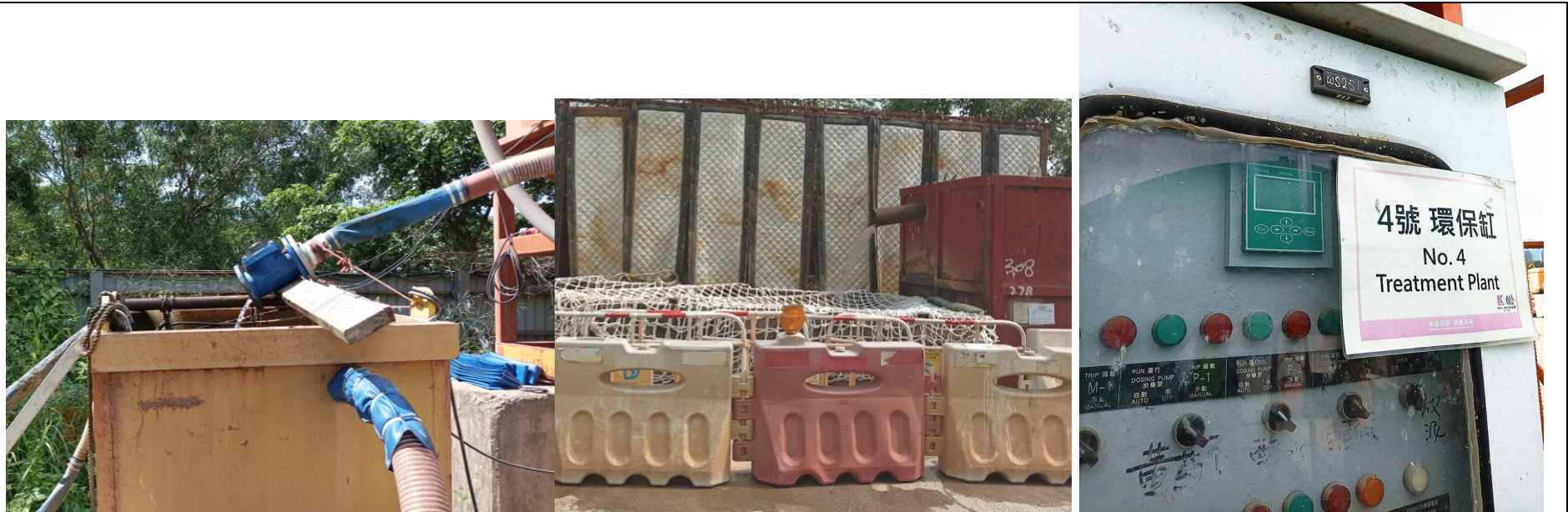
The site surface runoff was collected and directed to the sedimentation tank by the pump and properly treated in the treatment tank
